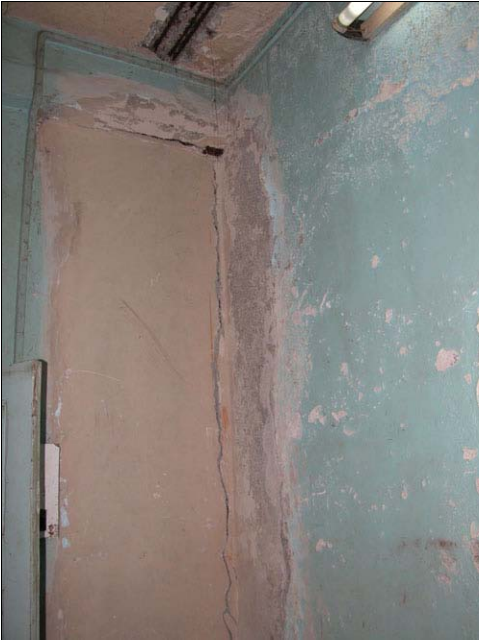
Figure 30 Masonry load bearing wall (S2-category)
