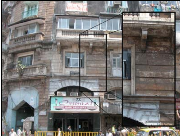
Figure 17 - Vertical crack in load bearing wall
