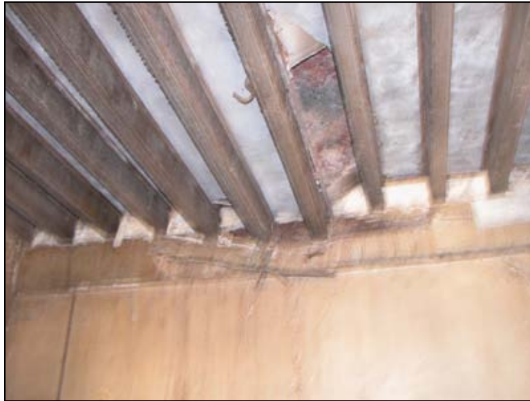
Figure 7 Weathering of timber joists at support
