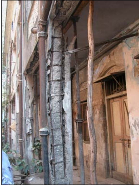
Figure 23 Spalling of cover concrete and buckling of reinforcement bars
