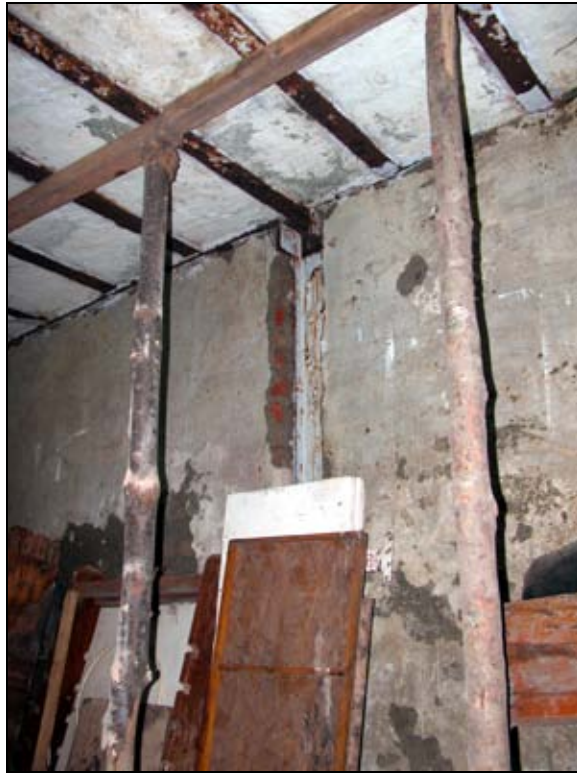
Figure 8 Rusting of steel joists (Only bottom flange is available for inspection)
