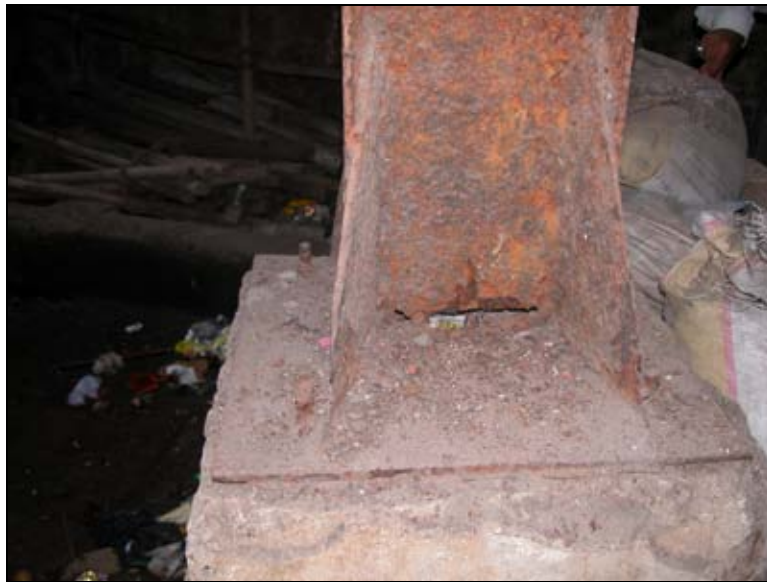
Figure 22 Reduced cross-section area of steel column
