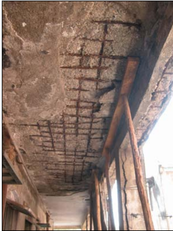
Figure 6 Spalling of slab cover concrete
