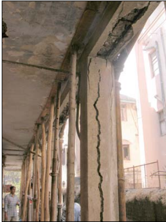
Figure 13 Concrete spalling at the bottom of beam because of tension
