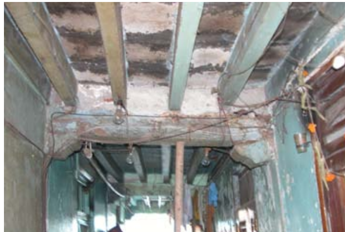
Figure 9 Sagging and support displacement of timber beam
