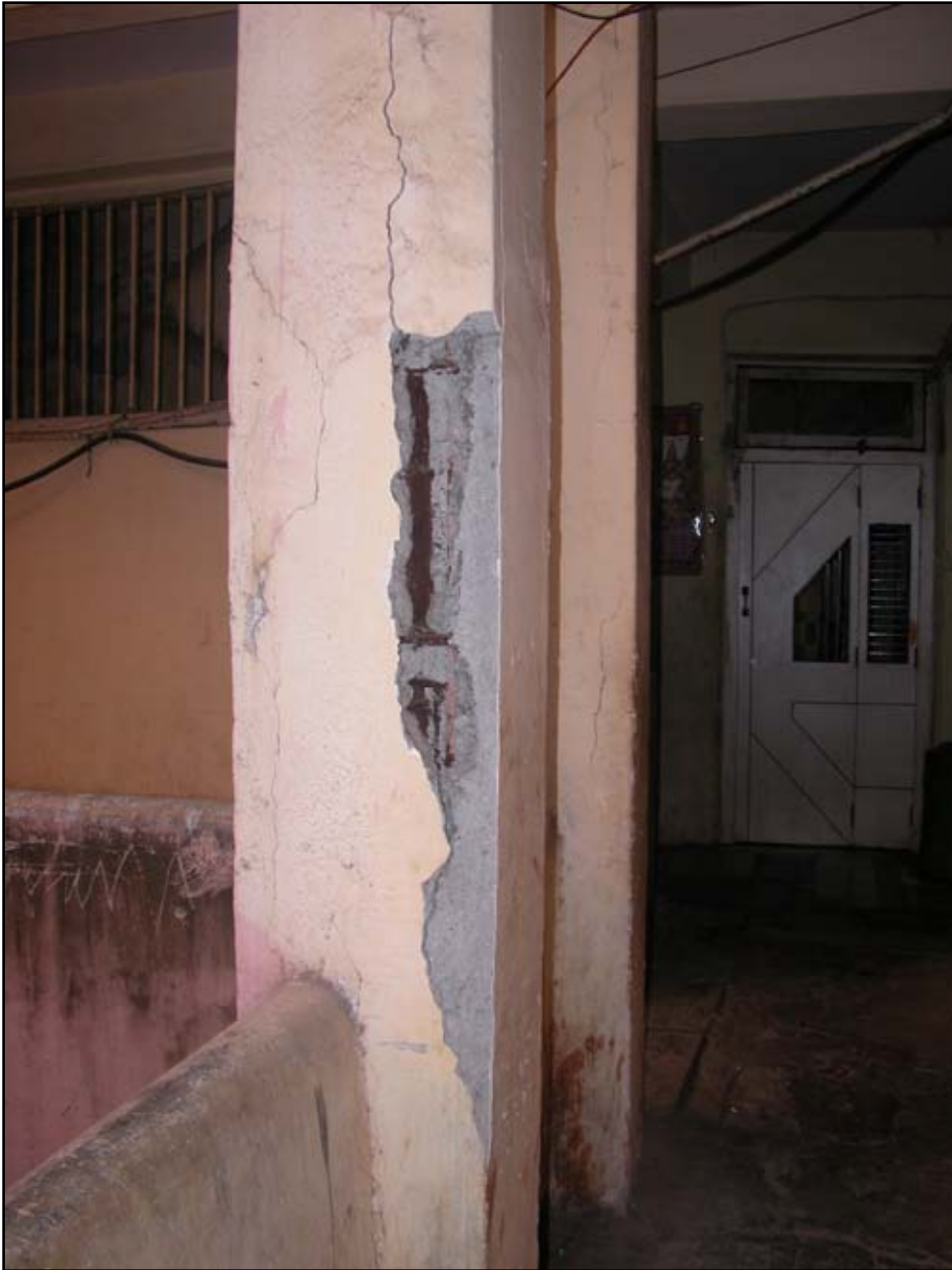
Figure 43 RCC column (S3-category)
