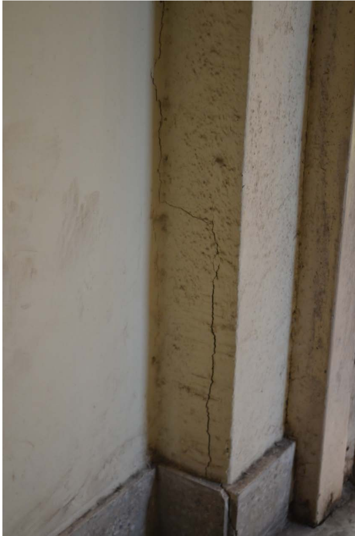
surface crack in concrete column
