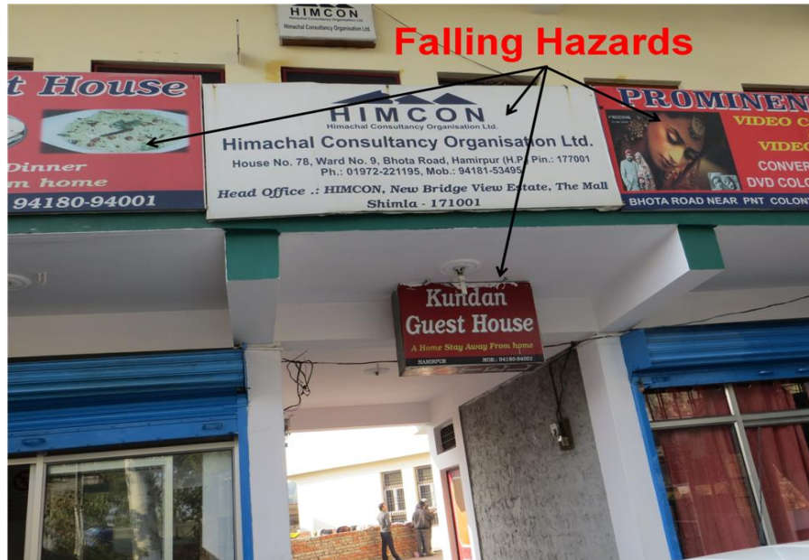
Figure 41: Falling hazards in a building
