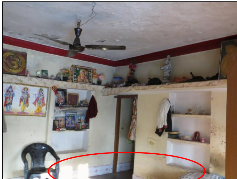
Figure 27: Water seepage problem in the roof and wall (Hamirpur, 16th December 2013)
