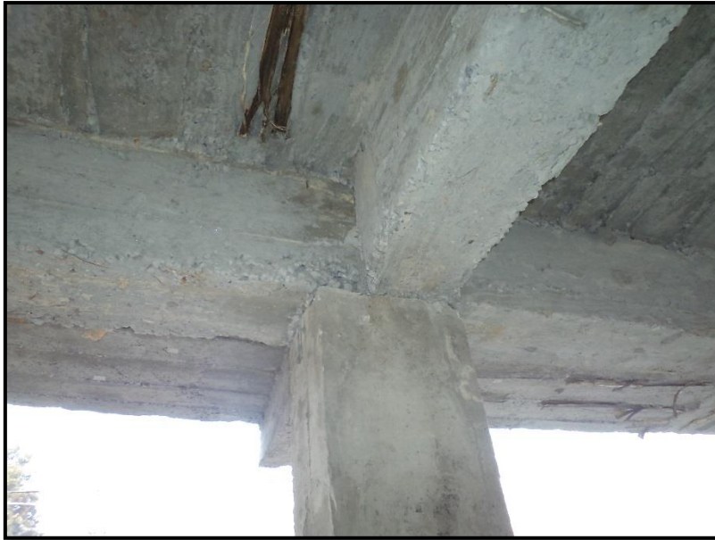
Figure 28: Wrong Practice of Beam Column Junction
