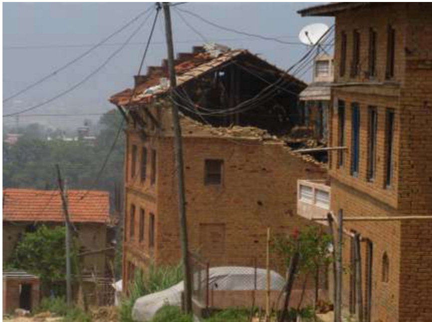
Collapse of the gable wall.
