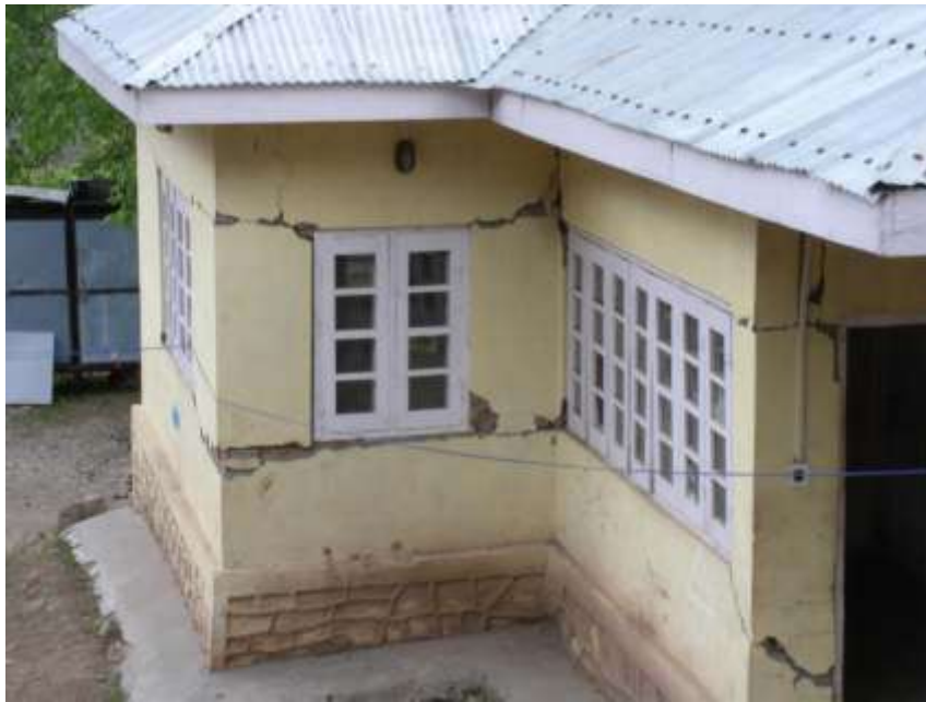
Diagonal cracks around openings
