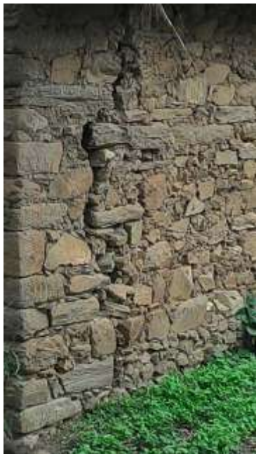
Separation of the wall from stone pier
