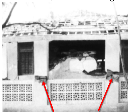
Masonry piers cracking
