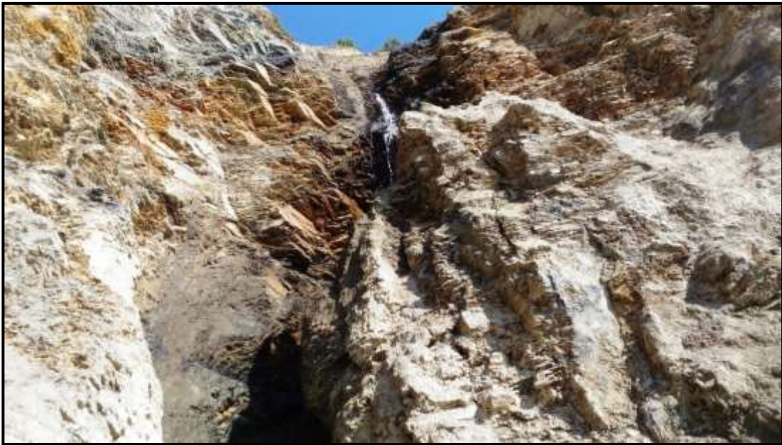
Fig.-4: Closer view of weathered and jointed slates exposed in sub-vertical scar.
