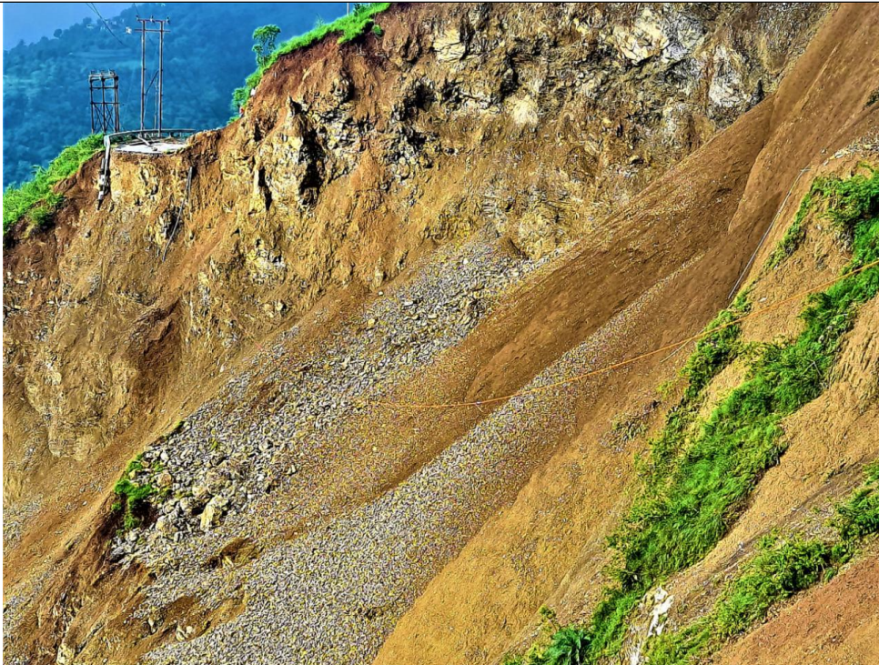
Fig.-6: Damage and complete wash out of 150m stretch of the NH-707 (View towards Sataun)
