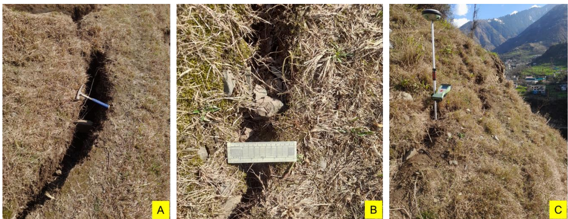
Photo 8. Representative photographs on the crack opening width and depth delineated at the right flank of the landslide.
