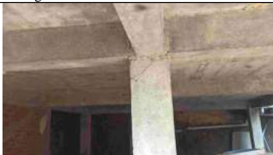
i. Cracks observed in the pillars of residential
