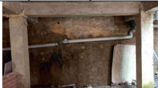
h. Seepage from the retaining walls of residential houses.
