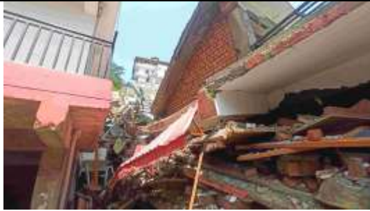
e. Collapsed RCC building
