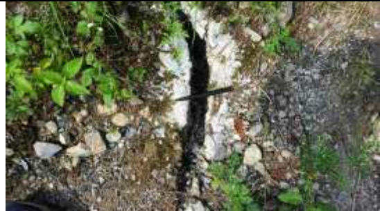
d. Ground cracks observed in Shamti area.
