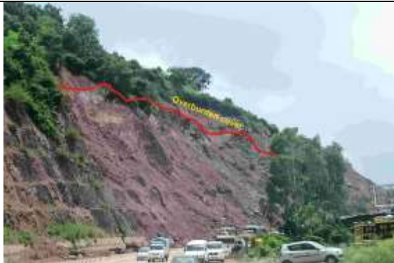
a. Thick overburden exposed in the vicinity of landslide.
