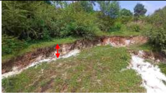
c. Ground subsidence observed at the crown portion
