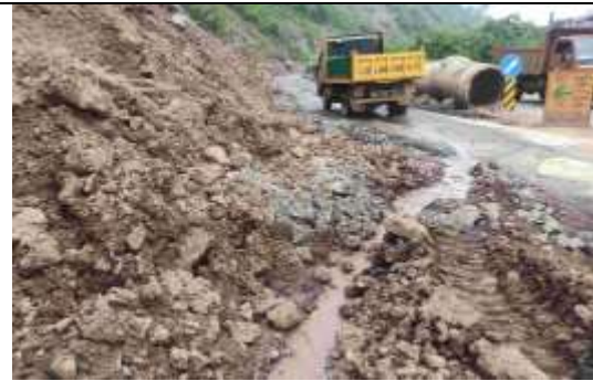
j. The flowing hydrological conditions observed along the road.
