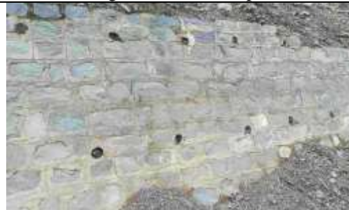
f. Chocked weep holes in the retaining walls along the road.
