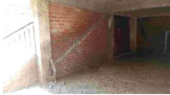
l. Cracks observed in the walls of residential houses.
