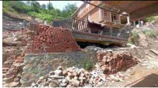
f. Collapsed RCC building
