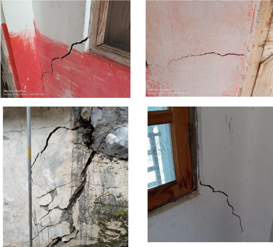
Fig. 52. Cracks due to differential settlement at various locations in building.
