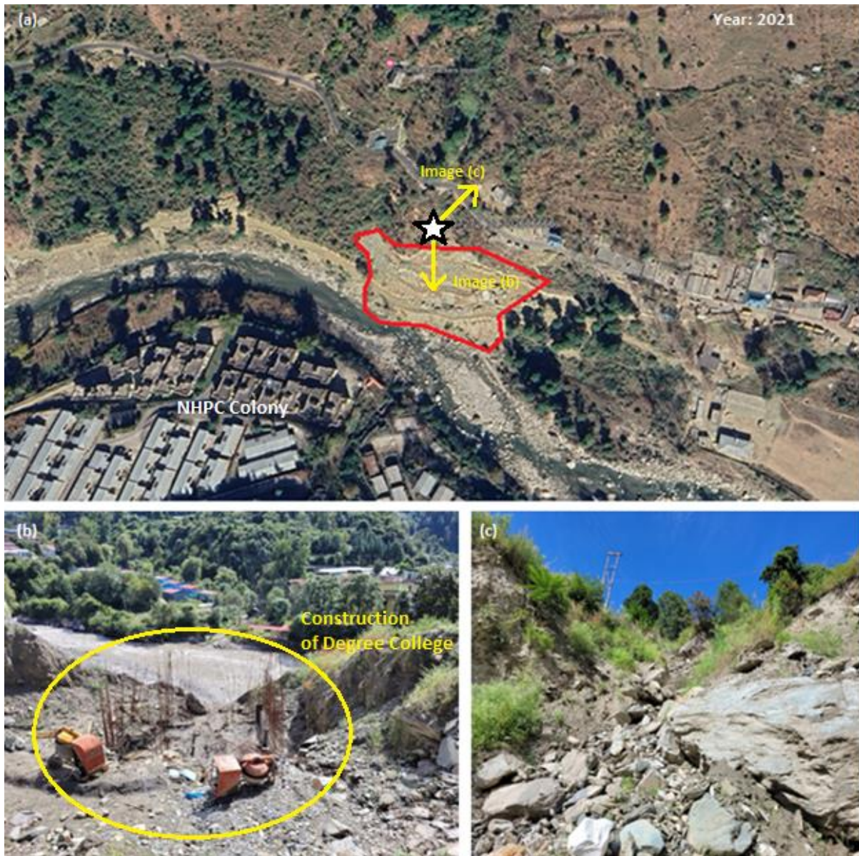
Fig. 19. Near the site for proposed Sainj Degree College, a 45-meter length of the road has been washed away. An adjacent landslide above the road led to collapse of retaining walls intended to provide slope stability.
