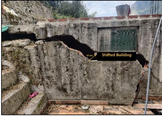
Fig. 28. Visible gap due to settlement of the building
