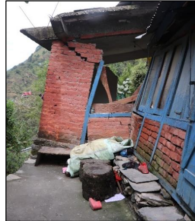
Fig. 15. Tilted house with large cracks.
