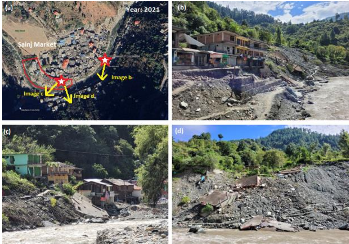
Fig. 17. Near Sainj Market, a landslide caused subsidence of ground by around 1.5 meters over a 50 meter area, resulting in displacement of the retaining wall intended to provide slope stability. The root zone stability of the orchards has been impacted.
