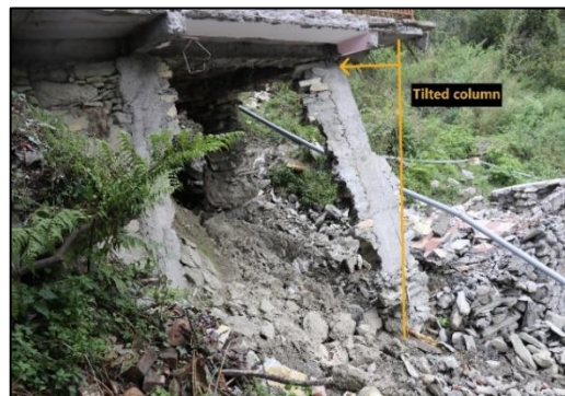
Fig. 38. Tilted column of school building.
