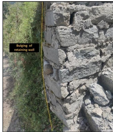
Fig. 31. Bulging of retaining wall.
