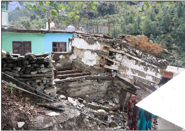
Fig. 24. Damaged house made of wood and stone.
