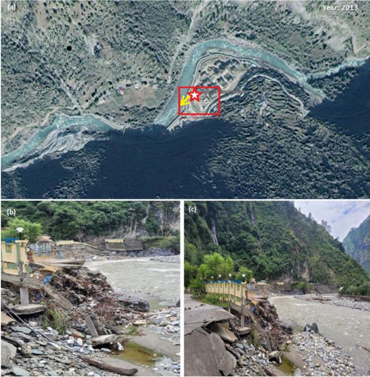
Fig. 13: Extensive damage to road infrastructure and collapse of retaining walls near NHPC residence at Spangani village caused by severe flash flooding. Major landslide visible on the opposite riverbank covering a span of around 100 meters.
