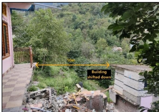
Fig. 37. Building shifted down due to subsidence.
