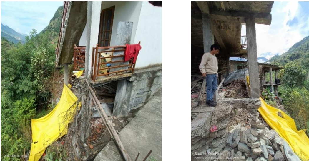
Fig. 51. Building collapse Kailash Niwas near Sharai
