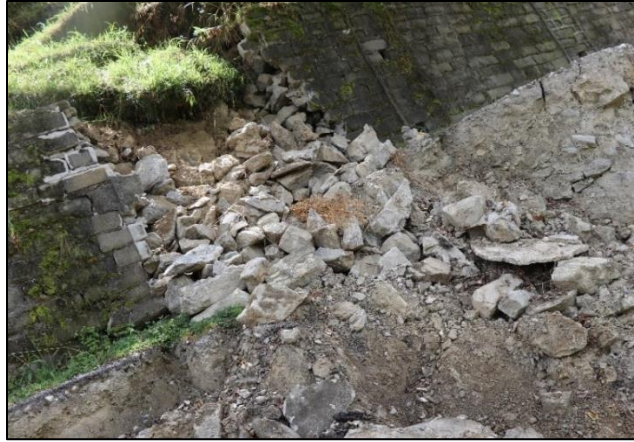
Fig. 32. Damaged retaining wall.
