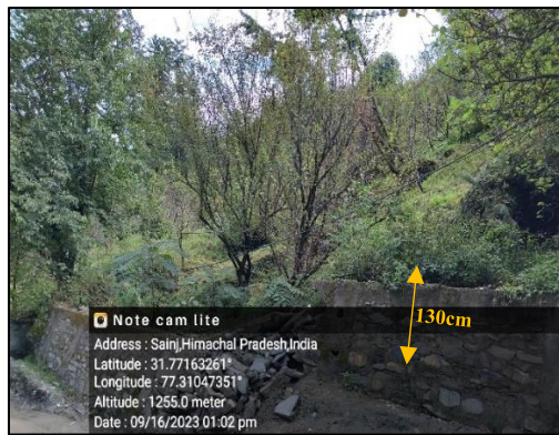
Fig. 43. Land subsidence, Sainj
