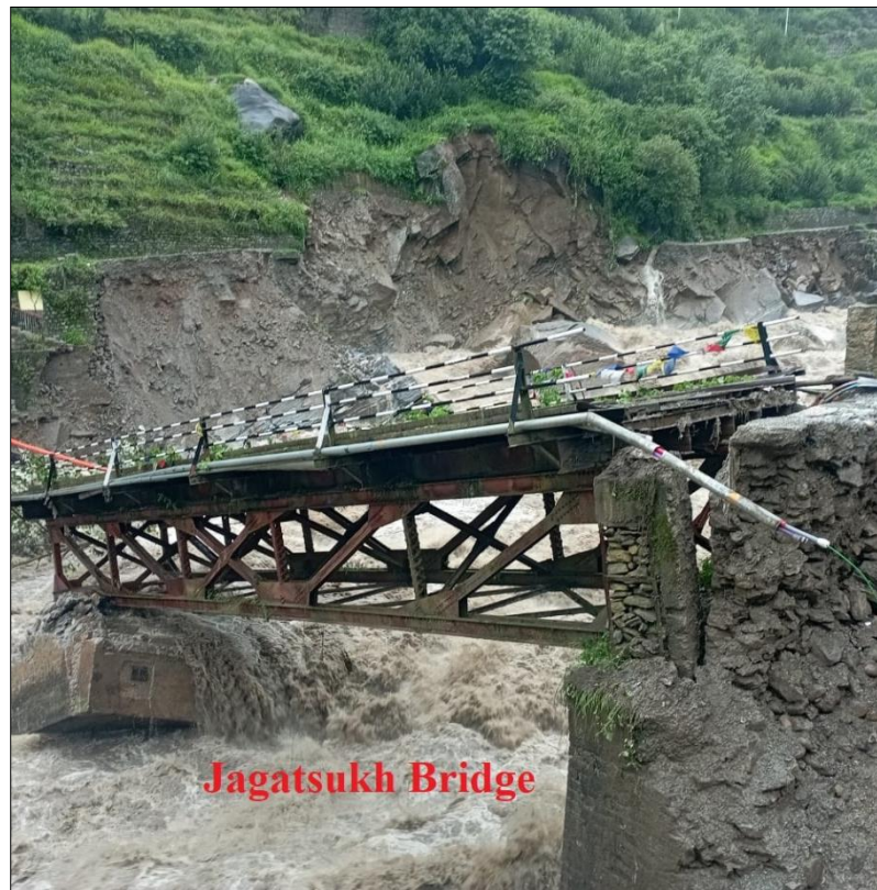
Fig. 61. Damaged Bridge located at Jagatsukh
