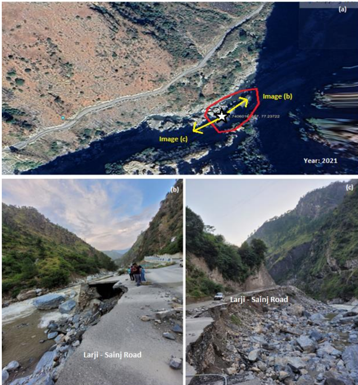
Fig. 23. In Bihali village, the paved road stretching approximately 300 meters constructed along the riverbank has been completely washed away due to flash floods eroding away the banks.
