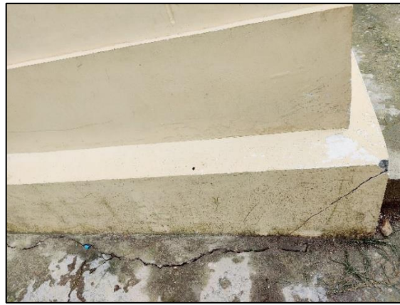
Fig. 36. Cracks developed in the newly constructed school building (just before monsoon).
