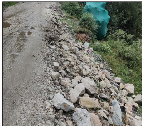
Fig. 27. Damaged Road filled with local material.
