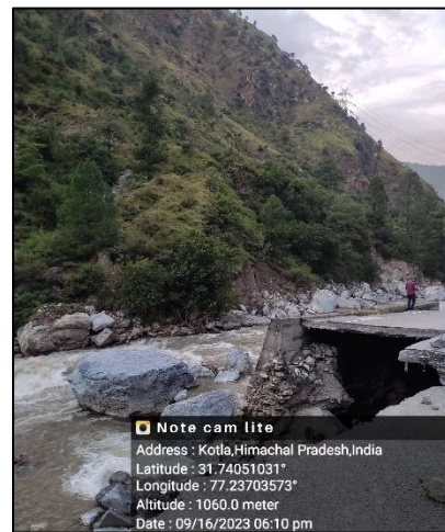
Fig. 50. Loss of pavement material due to erosion.
