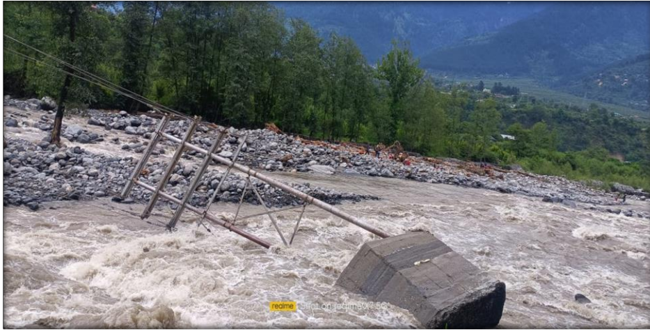
Fig. 62. Damaged Bridge located at Jagatsukh
