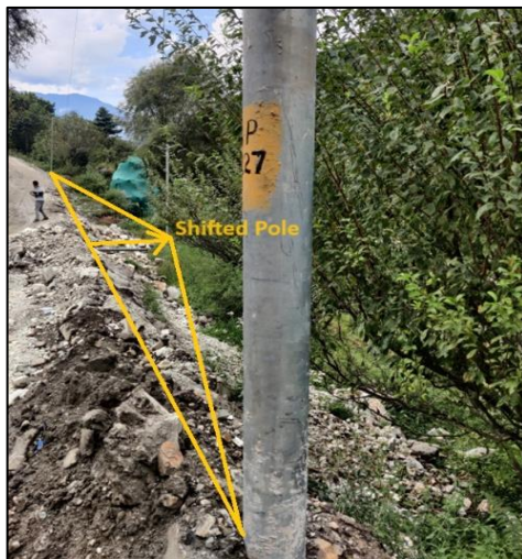
Fig. 26. Shifted pole due to subsidence.
