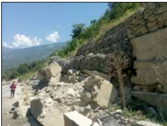
Fig.3; Damaged retaining walls towards the hill side along NH-3
