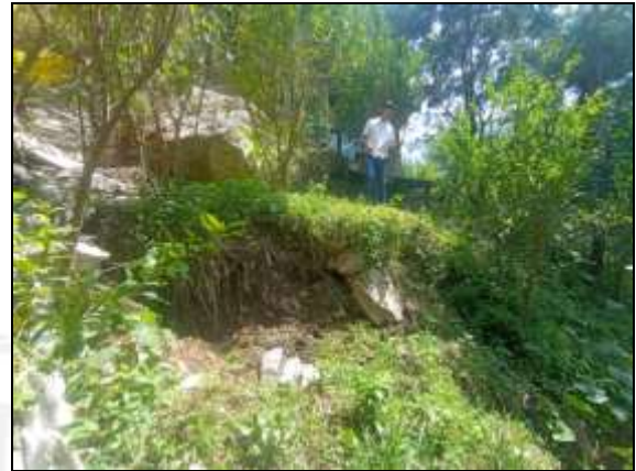
Fig.61; Ground subsidence below road at Sharai
