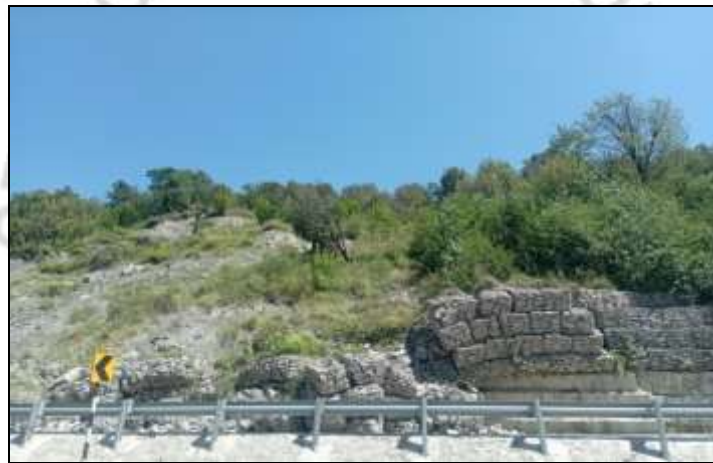
Fig.12; Damaged retention structures along the hill side of NH-3
