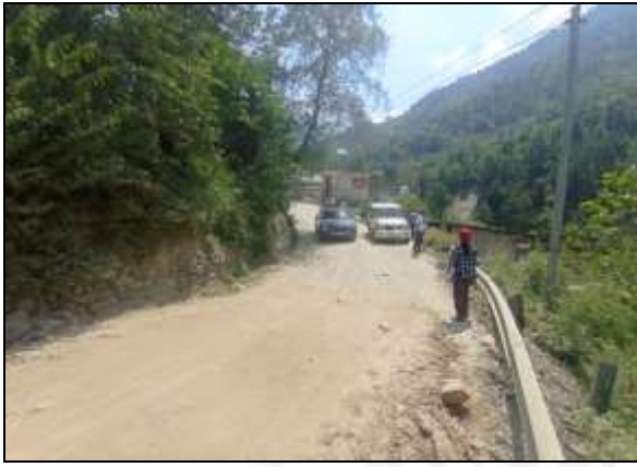
Fig.60; Road subsidence at Sharai
