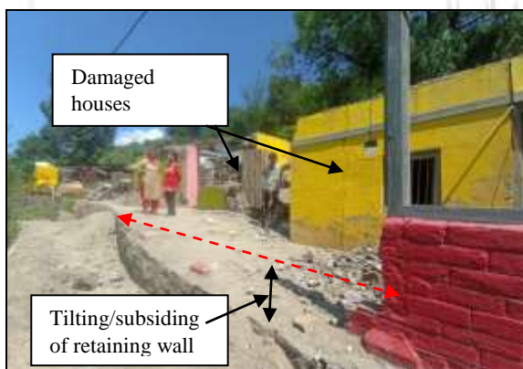
Fig.13; Damaged civil structures at Banontar Kharahal .
