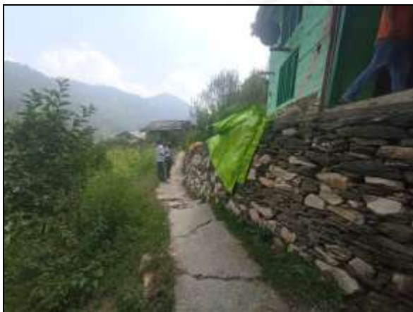
Fig.48; Ground cracks and partially damaged retaining wall.
