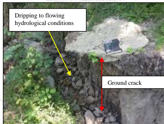
Fig.9; Seepage zone in flowing water conditions along ground cracks in the distressed slope.
