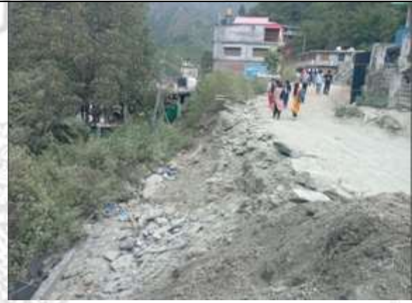
Fig.3. Damaged road stretch
