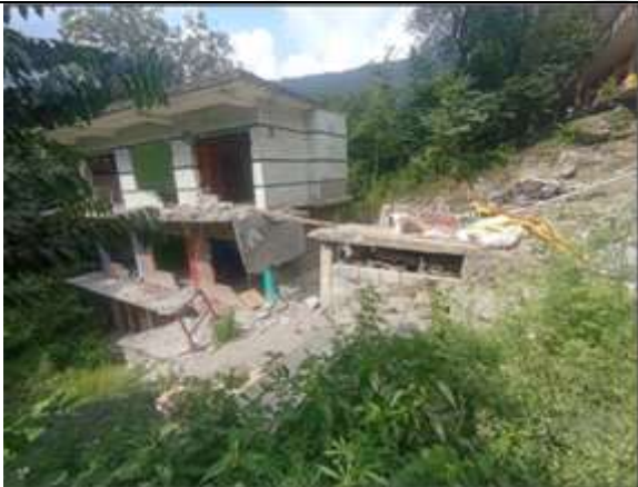
Fig.2. Damaged Sarswati Vidya Mandir Sr.Sec, School
