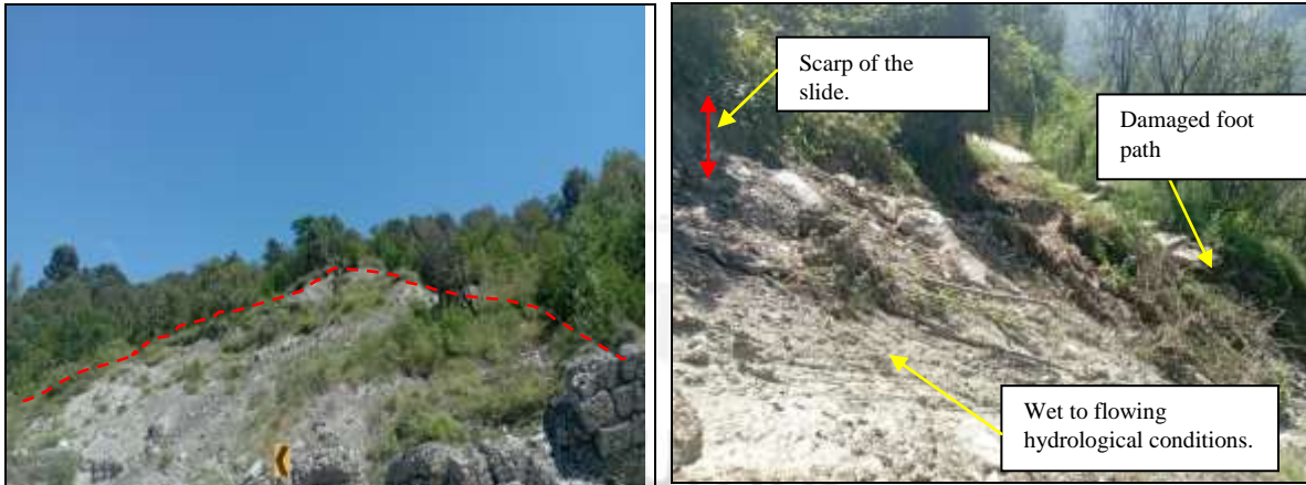
Fig.10; Debris slide as discernable from the left bank of Beas River. Fig.11; Main body of the landslide.
