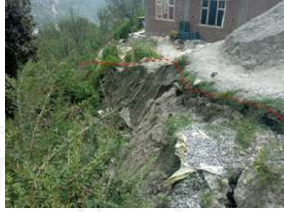
Fig.3. House at risk
