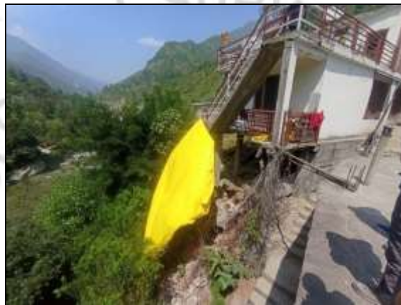
Fig.62; Damaged house present on the affected slope at Sharai.
