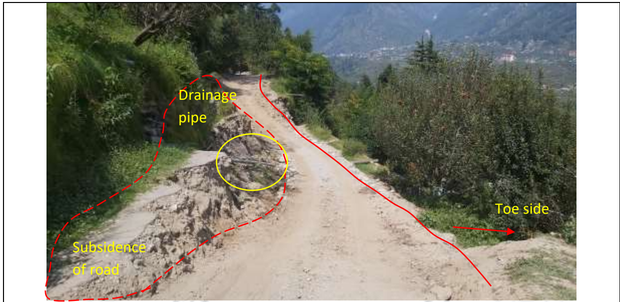
Fig.1. Subsidence of road observed in Shaleen village
