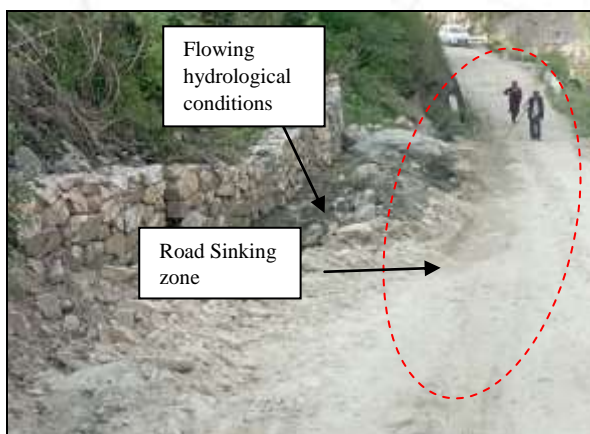
Fig.58; Road subsidence at Kartah
