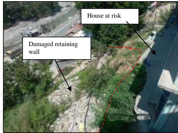
Fig.6; House at risk located upslope of NH-03 at Devdhar village.
