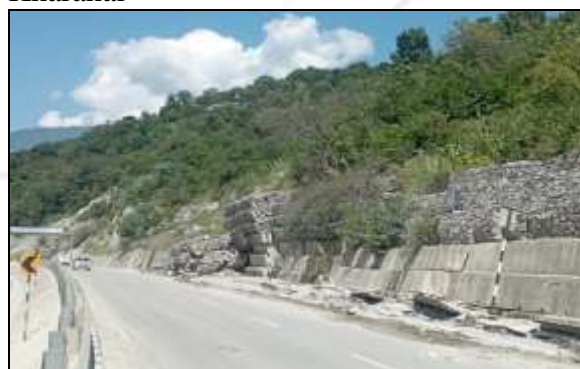
Fig.16; Damage retaining structures along NH-3 downslope of Banontar Kharahal .
