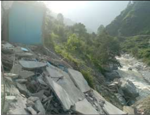
Fig.2. Damaged houses located near the bank of River
