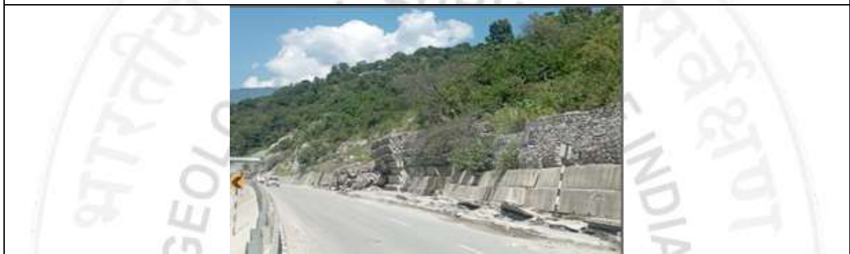
Fig.3 Damage retaining structures along NH-3.
