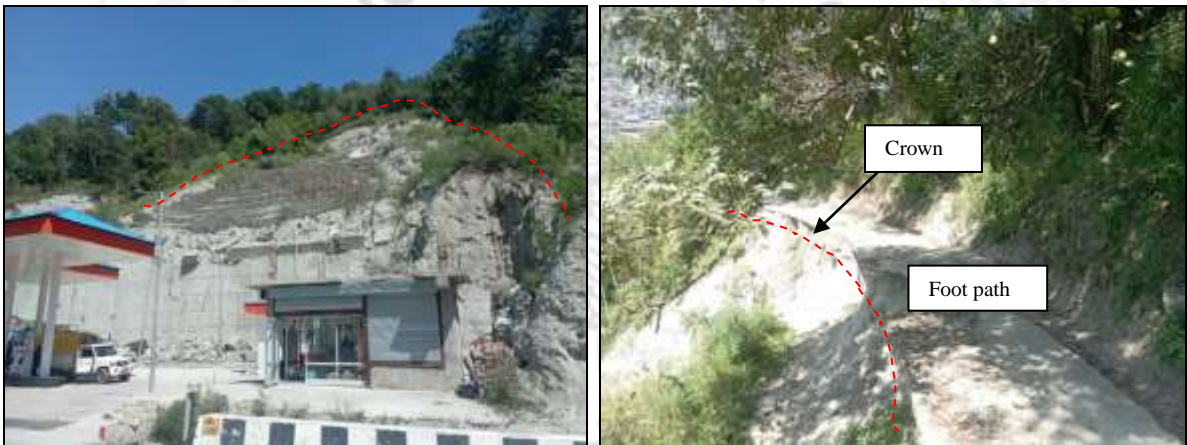
Fig.7; Debris slide on upslope of Indian oil petrol pump. Fig.8; Crown of the landslide.
