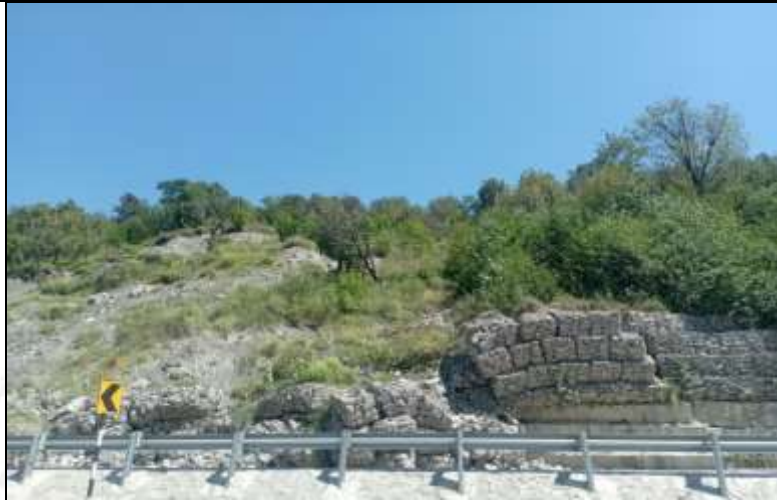
Fig.2. Damaged retention structures along the hill side of NH-3
