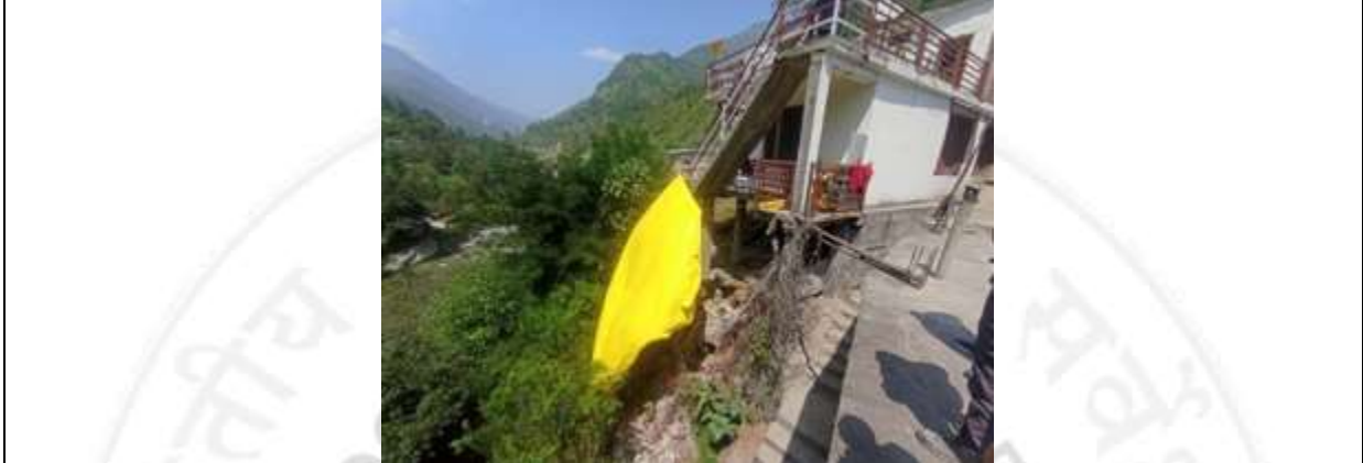
Fig.1.Damaged house present along the affected slope.
