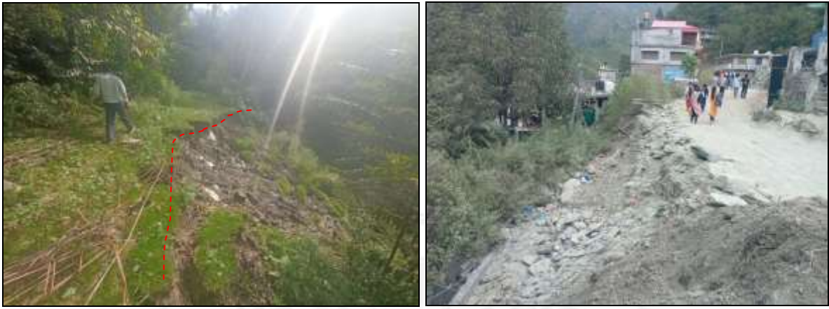
Fig.54; Dripping hydrological conditions on the distressed slope. Fig.55; Damaged road stretch at Daduhar.
