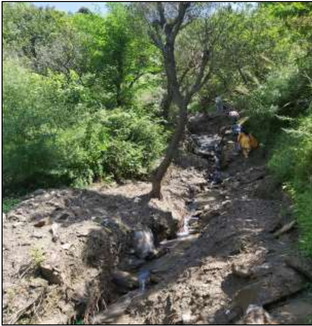
Fig. 64. Flowing nala observed near the Rageli slide
