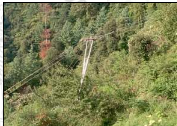
Fig.20; Tilting of electric pole located near seasonal Nala on the right flank of Garsa village.
