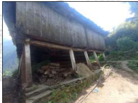
Fig.24; Tilting of houses at Barauna village.
