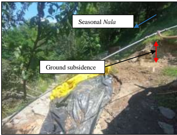
Fig.5; Ground subsidence observed along the left flank/ slope of seasonal Nala
