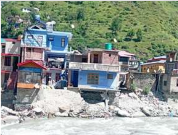
Fig.2. Houses at risk (Right bank of the river)
