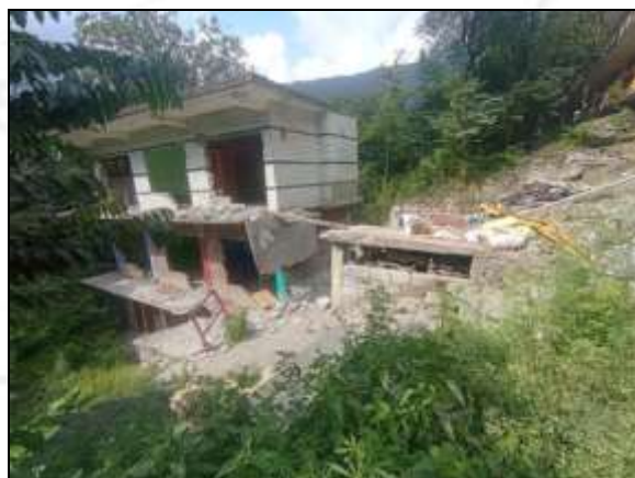
Fig.53; Damaged Sarswati Vidya Mandir Sr.Sec, School at Daduhar.
