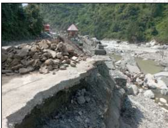
Fig.40; Severe road damaged near Thana Sainj.
