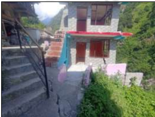
Fig.23; Crack on civil structures at Barauna village
