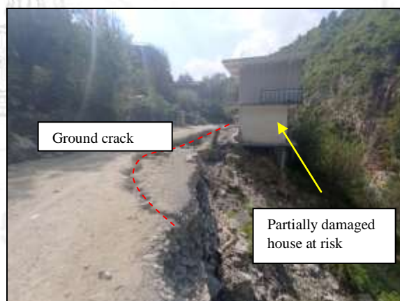
Fig.41; Ground cracks and House at risk located towards valley side of the road along Thana Sainj to Taxi stand road stretch.
