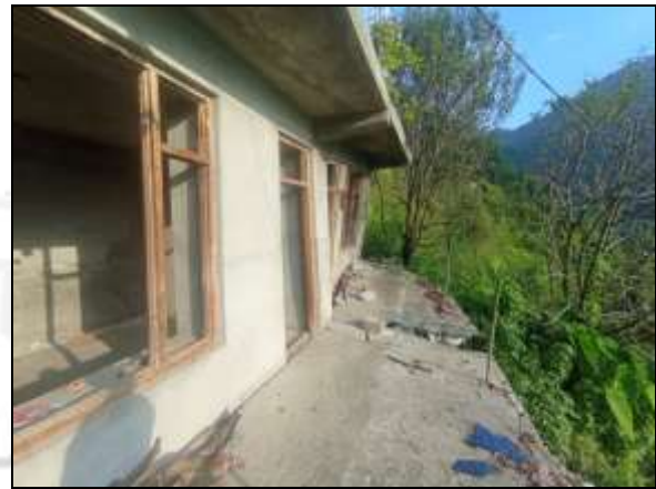
Fig.18; Damaged house at Garsa village.
