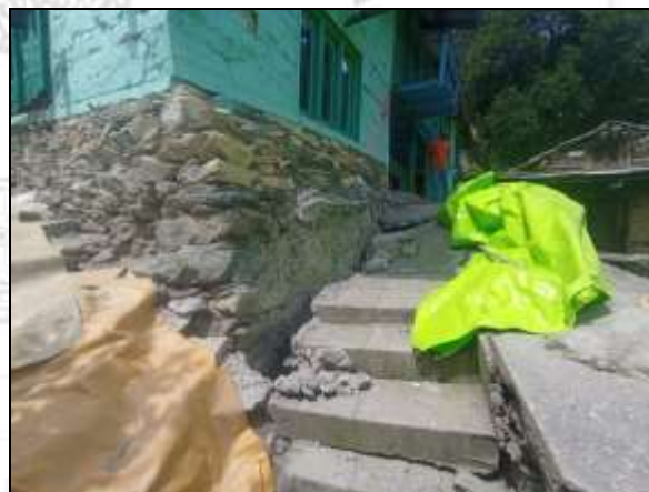
Fig.51; partially damaged houses Mourod
