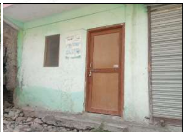
Fig.59; Cracks on walls at Kartah.
