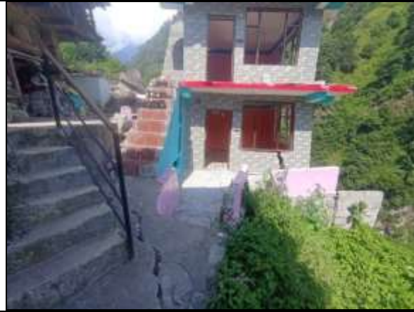
Fig.2. Crack on civil structures
