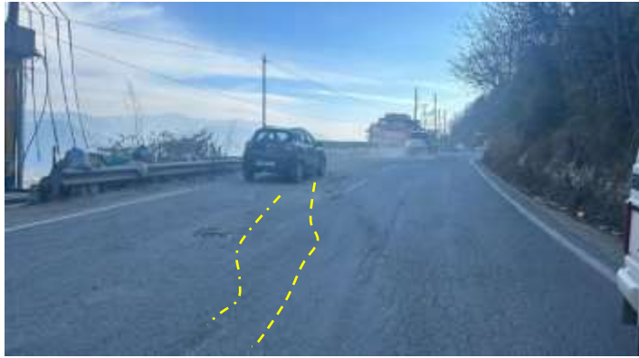
Ground cracks along Road at Himfed Petrol Pump
