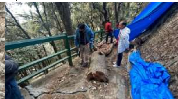
f. Cracks along the pedestrian pathway
