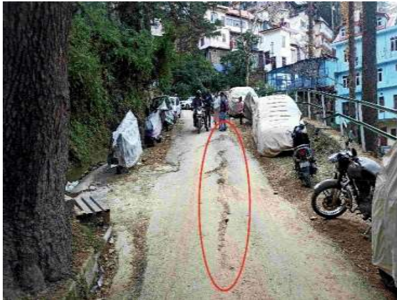
c) Longitudinal cracks on Comely Bank Road.
