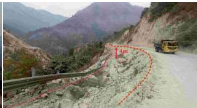
f) Ground subsidence along the NH-05
