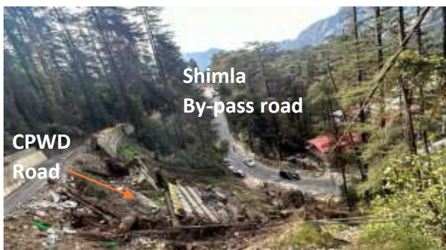
Figure 8 (d) Damaged CPWD road and retaining structures
