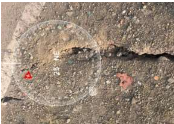
Figure 6 (e) Ground cracks trending N25° E at Dimple Dhaba
