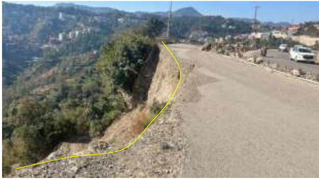
Figure 12 (b) Road cave in at Mohan Mekin Landslide, Solan Dist. Himachal Pradesh.
