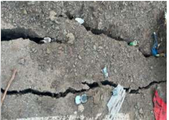
Figure 6 (h) Ground cracks trending N20°E at Haveli
