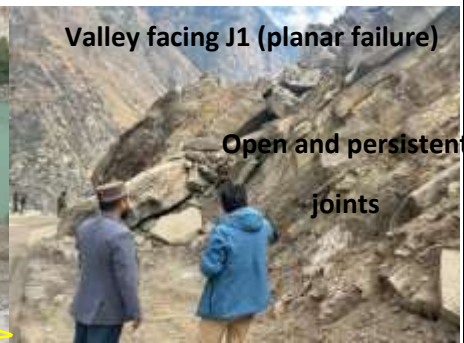
Open and persistent Valley facing joints
