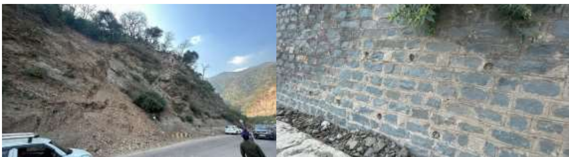
Figure 5 (f) Loose overhanging blocks on the upslope of Datyar slide
