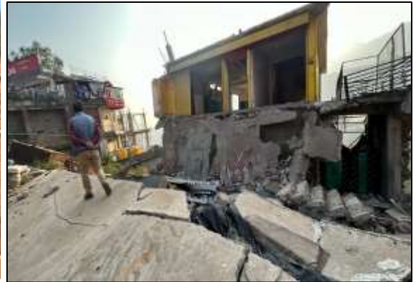
Figure 6 (d) Collapsed building due to subsidence
