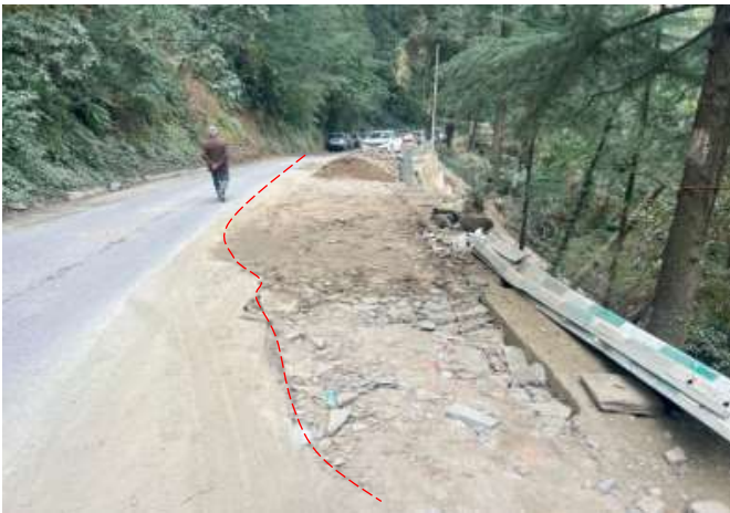
Figure 11(c) Subsidence observed along road section
