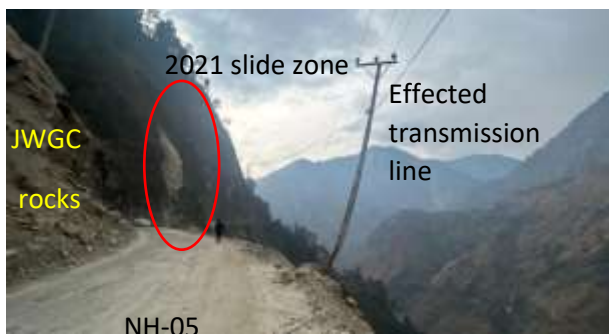
Figure 23(a) Highly jointed rocks of Jeori Wangtu Gneissic complex loosely hanging over National Highway-05 near old slide zone of 2021.
