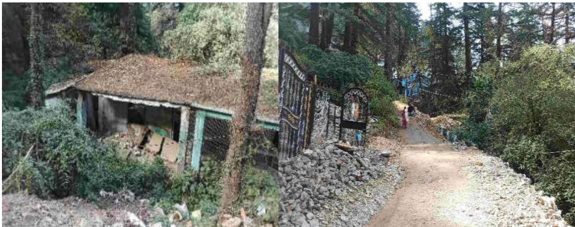
a) Damaged school building along the Comely Bank Road. b) Stretch of damaged Comely Bank Road.
