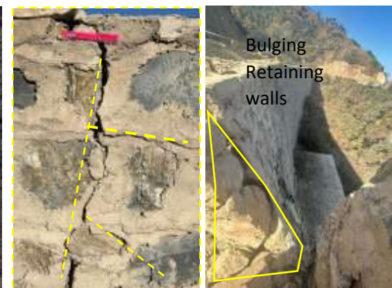
Figure 13 (d) damaged ( bulging and cracks ) retaining wall at Mansar, Solan Dist. Himachal Pradesh showing wide open cracks
