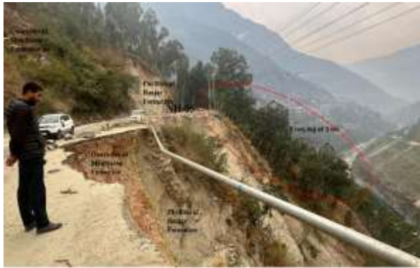
Figure 19 (a) Road cave in near Khaneri Hospital, Nogli, Rampur
