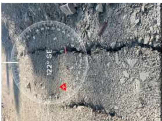
Figure 13 (c) wide open cracks trending 122° SE.
