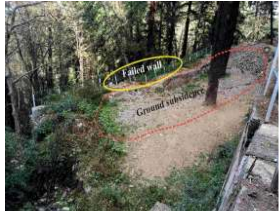
d) Ground subsidence and failed wall at parking area.
