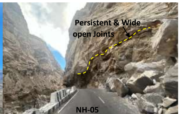
Figure 26(d) Wide open and persistent cracks at NH-05, Kinnaur
