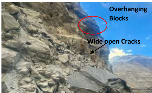
Figure 26(c) Wide open cracks and overhanging blocks at NH-05, Kinnaur
