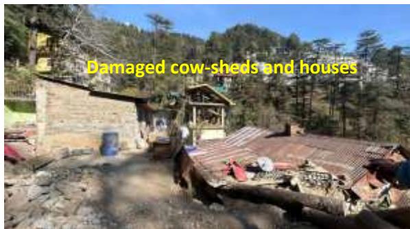
Figure 7 (c) Damaged houses and cowsheds located on 1 st order stream highly susceptible to future slide
