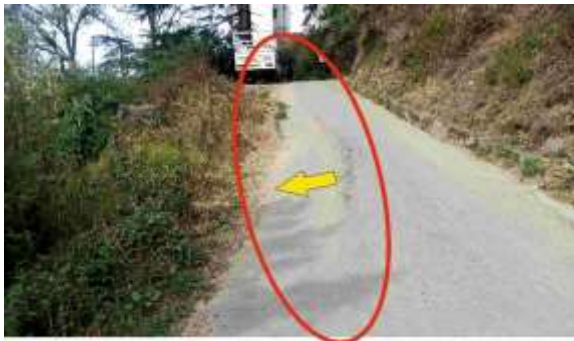
i) Subsidence observed along the Comely Bank Road.
