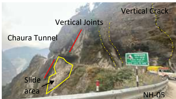
Figure 23(c) Vertical open joints with cracks near Chaura tunnel.
