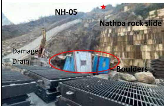
Damage to SJVNL dam
