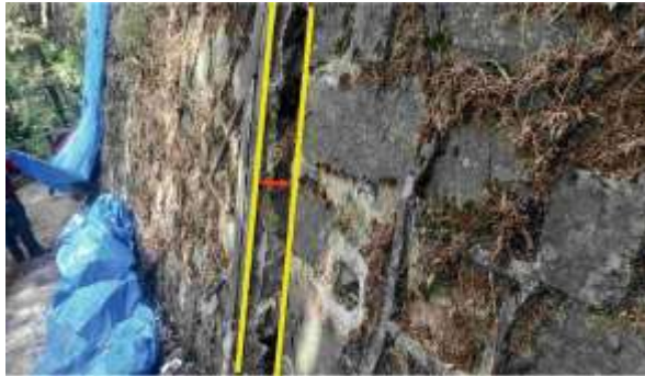
c. Displaced retaining wall along the failed slope.
