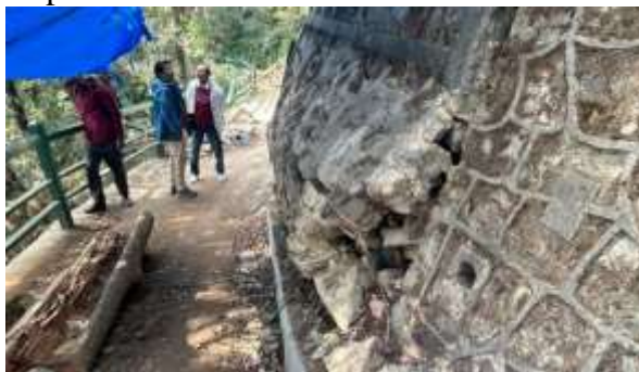
e. Bulged retaining walls along the pedestrian pathway
