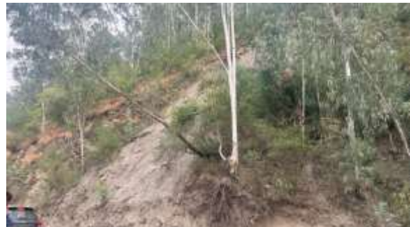
Figure 18 (d) Minor slide in upslope of slide zone showing creeping movement of trees.
