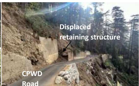
Figure 8 (e) Displacement of the retaining wall by 2 m along CPWD road
