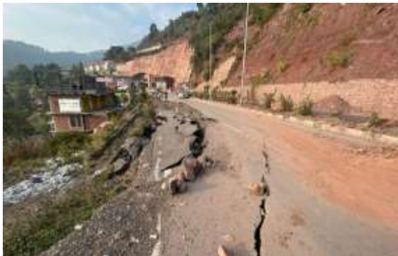
Figure 6 (a) Ground cracks along NH-05 near collapsed Dimple Dhaba.
