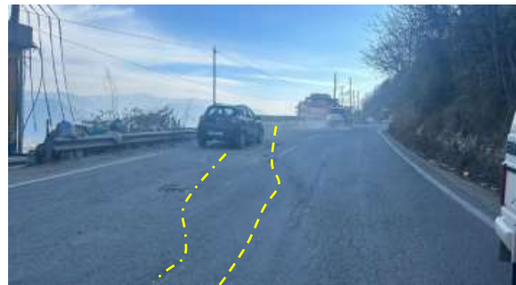
Figure 16 (b) Ground cracks along Road at Himfed Petrol Pump
