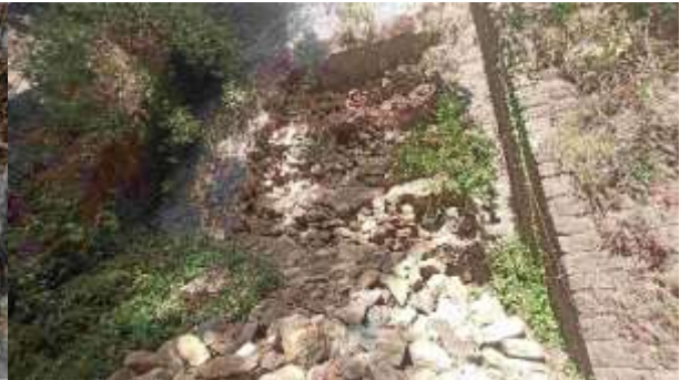
d. Partially covered wall along the failed slope.
