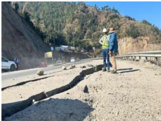
Figure 13 (a) Subsiding National Highway at Mansar, Solan Dist. Himachal Pradesh showing wide open cracks
