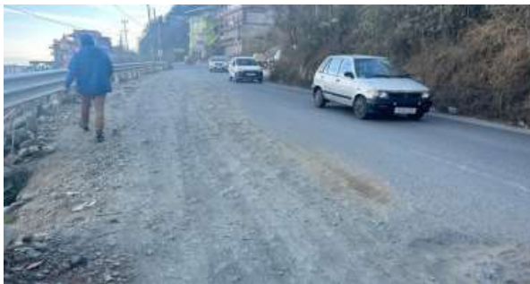
Figure 16 (a) Road subsidence at Himfed Petrol Pump
