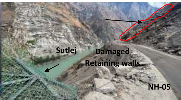
Figure 25(c) Toe of Nathpa Rock Slide, Kinnaur District, Himachal Pradesh
