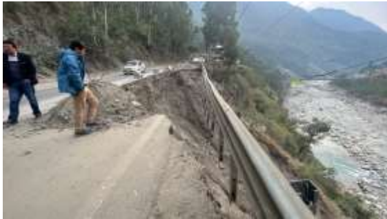
Figure 18 (a) Road cave in near Hyundai Showroom, Nogli, Rampur
