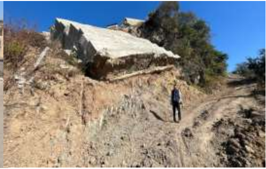
Figure 12 (c) Damaged retaining structure and road to PHC, Summer hall, Solan
