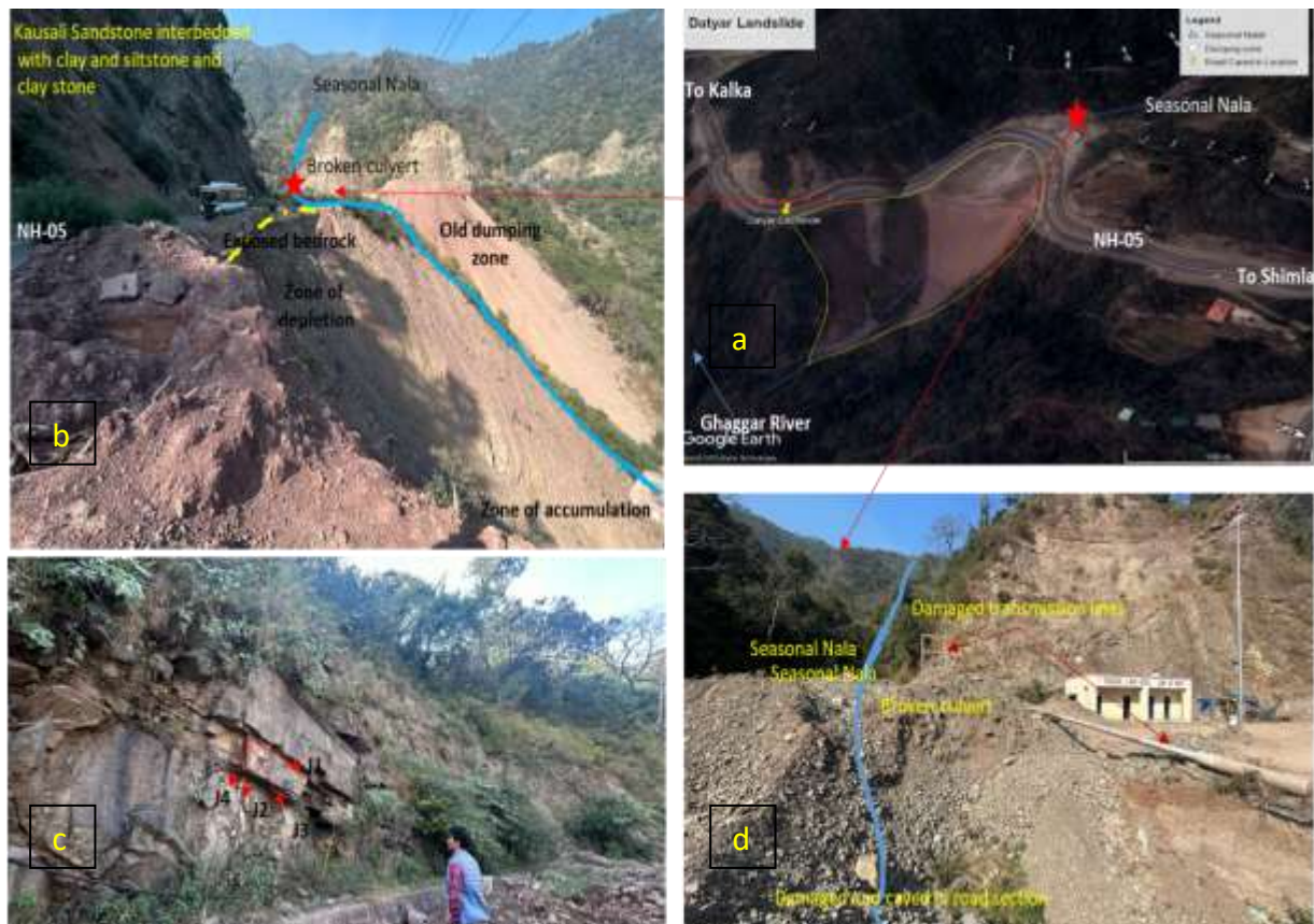
Figure 5(a) Morphometry of the Datyar Landslide, 5(b) Satellite imagery of Datyar landslide along NH-05 , 5(c) 3 set of prominent joint and one set of random joints along the sandstone of Kasauli Formation, 5(d) Seasonal Nala cutting across road causing major damage.
