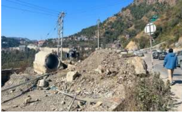
Figure 12 (g) Damaged culverts and transmission lines at Mohan Mekin Landslide, Solan Dist. Himachal Pradesh.
