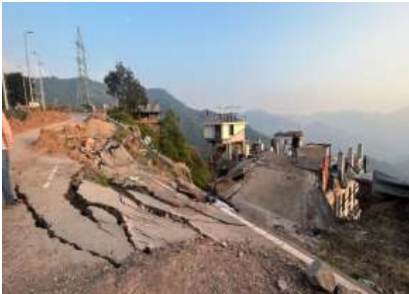
Figure 6 (g) Damaged AAA hotel due to subsidence
