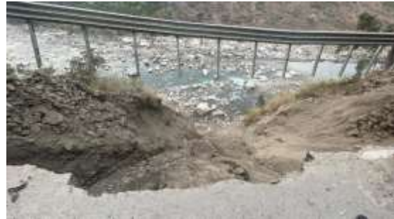
Figure 18 (b) Gully erosion and toe cutting action of Sutlej River
