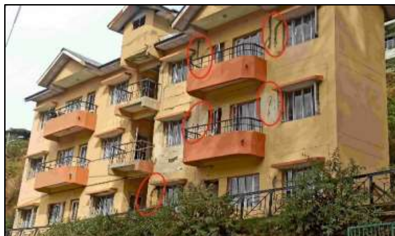
g) Damaged buildings along the Comely Bank Road.
