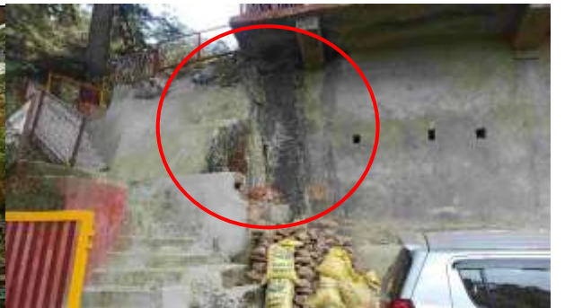
h) Cracks at the foundation level in residential building along the road.
