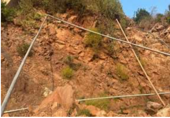
Figure 6 (c) Highly Jointed sandstone on upslope of NH-05
