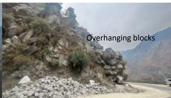
Figure 23(b) Highly jointed rocks of Jeori Wangtu Gneissic complex loosely hanging over National Highway-05 near Chaura tunnel.
