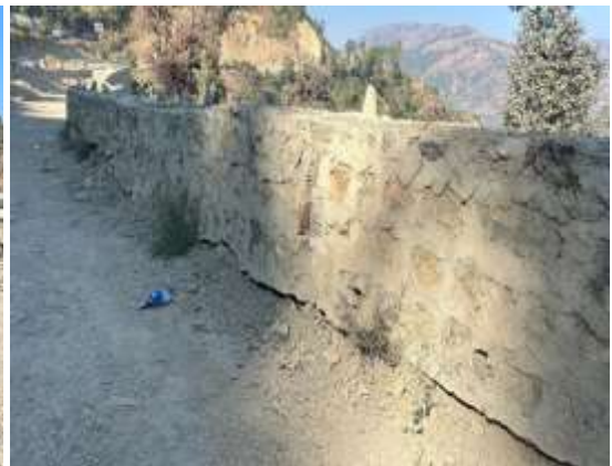
Figure 13 (b) damaged foundation of retaining wall at Mansar, Solan Dist. Himachal Pradesh showing wide open cracks
