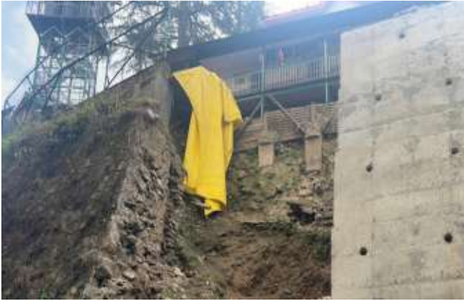
Figure 11(a) Damage to the foundation of the house and retaining wall
