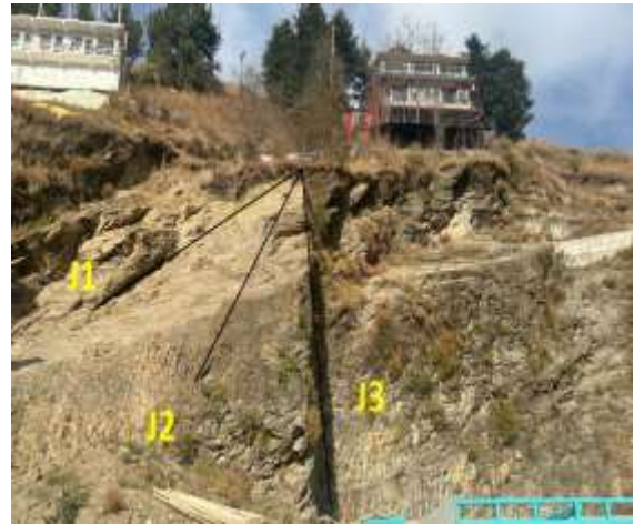
Figure 15 (c) Highly jointed slates of Basantpur Formation showing three set of prominent joints
