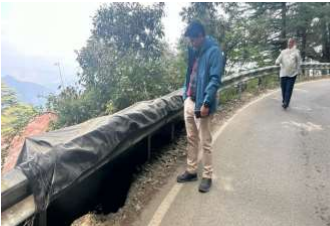
Figure 11(e) Minor slides observed along road section
