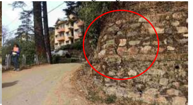
j) Cracks observed in the retaining wall along the road.
