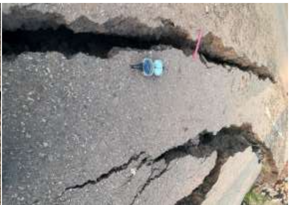
Figure 6 (f) Ground cracks trending N230° at AAA hotel
