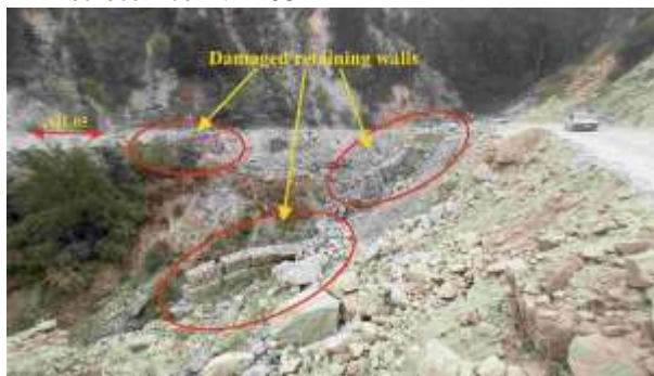
g) Failed retaining structures along the NH-05
