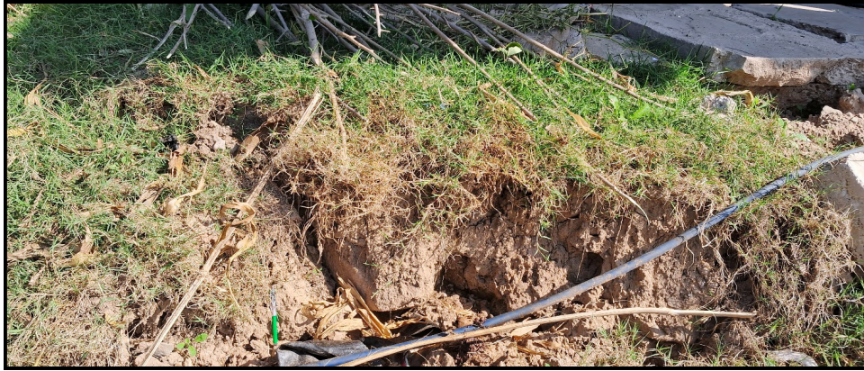
Fig. 19: Traces of ground cracks (next to temporary drain) as observed in strike continuity of Mahila Mandal Complex at Jabbal Village.
