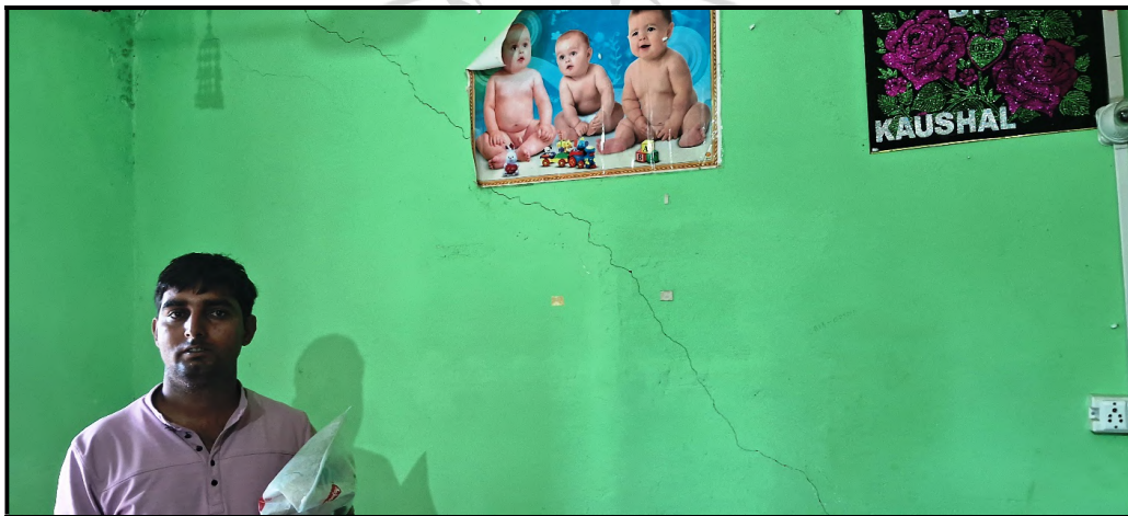
Fig. 32: Presence of crack in house(s) located on valley side, in the immediate upslope of Samthana slope failure.
