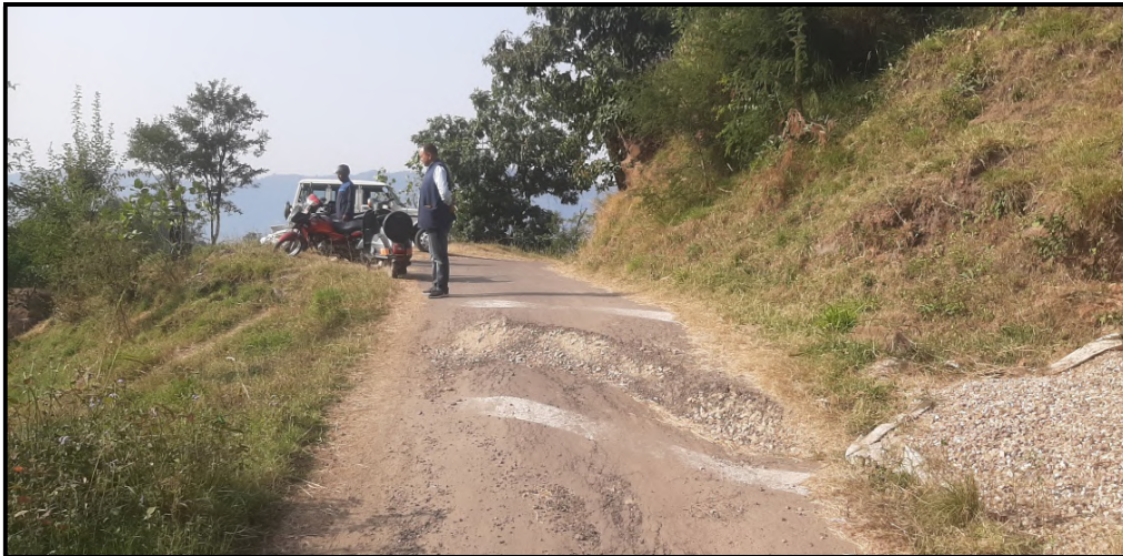
Fig. 22: A relatively smaller subsidence incidence as observed along approach road of Khairian Village.
