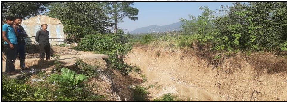
Fig. 04: Proximal view of the major gully (~ N160° to N210°), as observed along right bank of Sukar Khad (Note the partially damaged civil structure along right bank).
