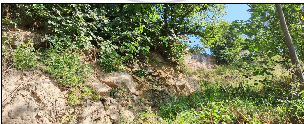
Fig. 28: Outcrops of weathered and jointed sandstone rock mass were observed towards right fringe of the failure.
