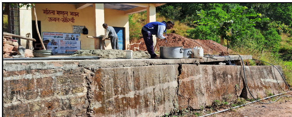
Fig. 16: Instability signatures (damage to skirt wall: Note the right portion of the Fig.) as observed in Mahila Mandal Complex, Jabbal Village.
