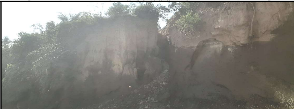
Fig. 12: Weathered and jointed rock mass and widened joint(s) towards u/s end of major gully, as observed along right bank of Sukar Khad .
