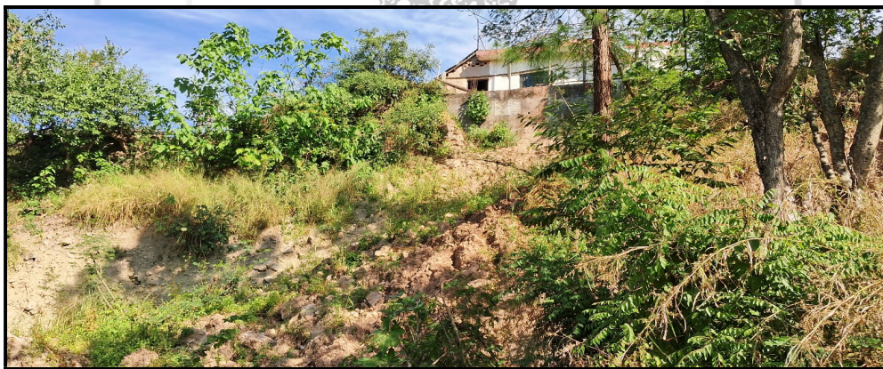
Fig. 27: Proximal view of Samthana Slope failure incidence
