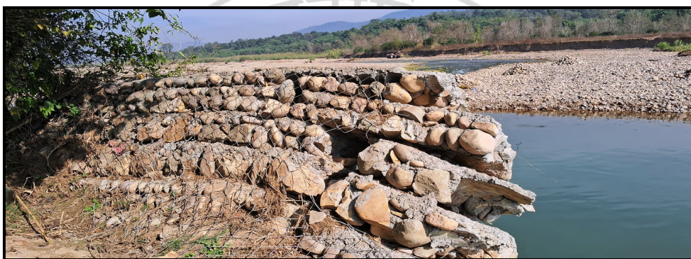
Fig. 14: Partly tilted and damaged retention structures seen along right bank of Sukar Khad .
