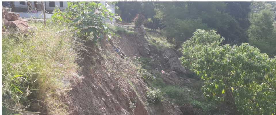
Fig. 21: Minor slope failure that took place in further strike continuity of Mahila Mandal Complex.
