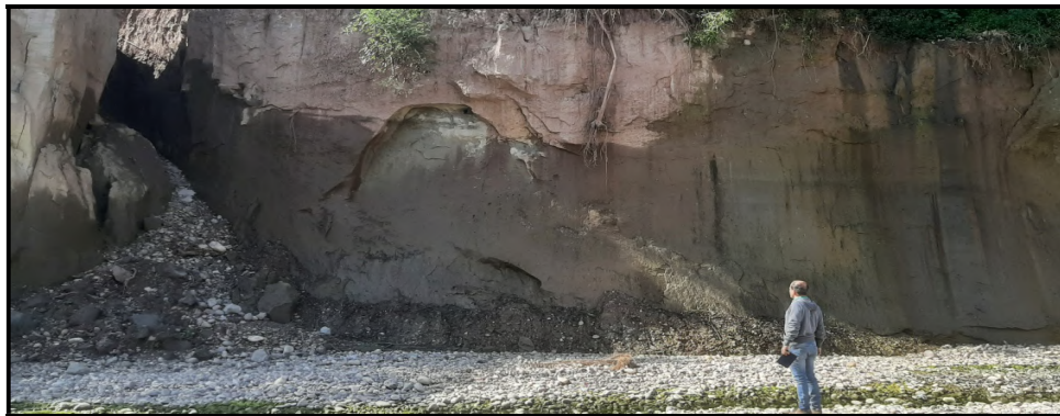
Fig. 11: Weathered and jointed rock mass exposed towards u/s end of the major gully, as observed along right bank of Sukar Khad .
