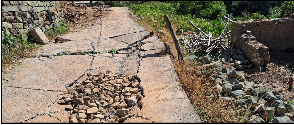
Fig. 17: Instability signatures (damage to dry stone wall and foot track) as observed in Mahila Mandal Complex, Jabbal Village.
