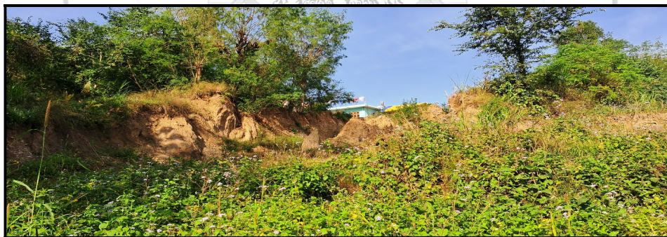
Fig. 05: Proximal view (as observed in d/s side) of the major gully, as observed along right bank of Sukar Khad (Note the partially damaged civil structure along right bank).
