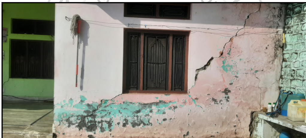
Fig. 23: Crack observed along one wall of a house, located along the agriculture terraces built up within house premises.
