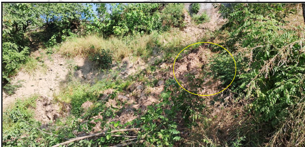
Fig. 29: Presence of ground cracks within failure zone (Indicated by Yellow oval)
