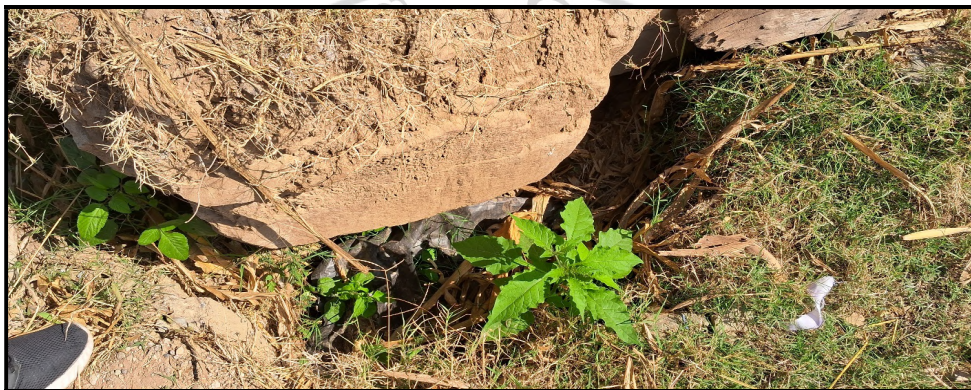
Fig. 20: Traces of ground crack below a sandstone rock mass outcrop (?) as observed in strike continuity of Mahila Mandal Complex at Jabbal Village.
