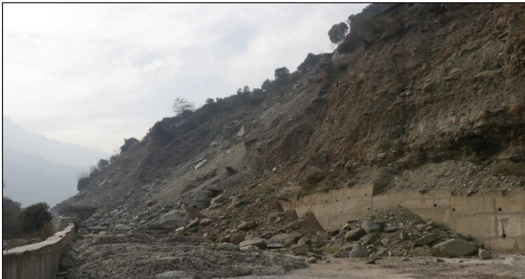
Landslide at site 2 (right view).
