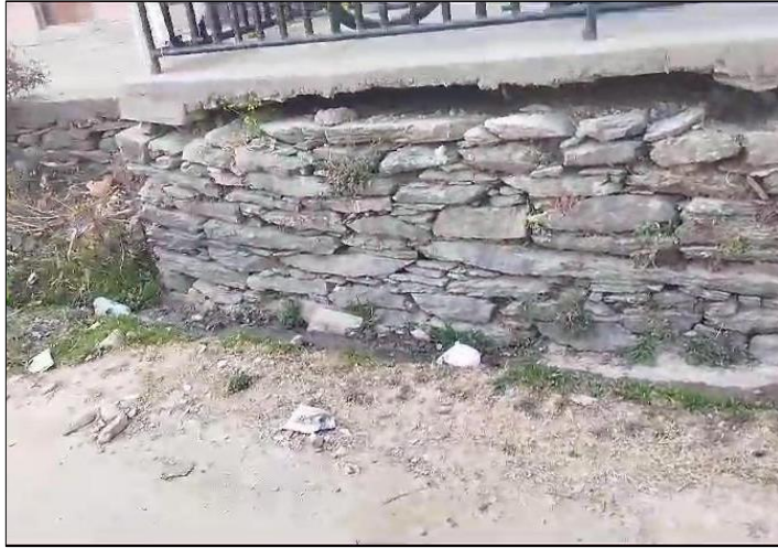
Settlement in house.
