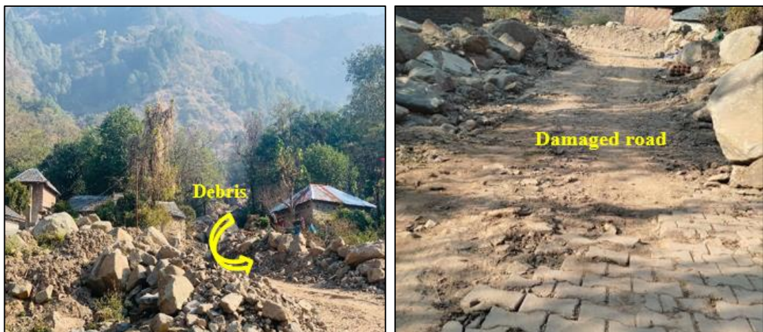
Damage due to Debris flow.
