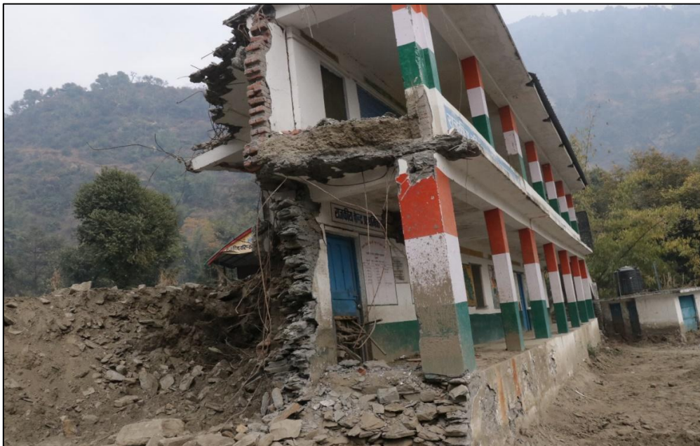
Damaged Govt. School Building.
