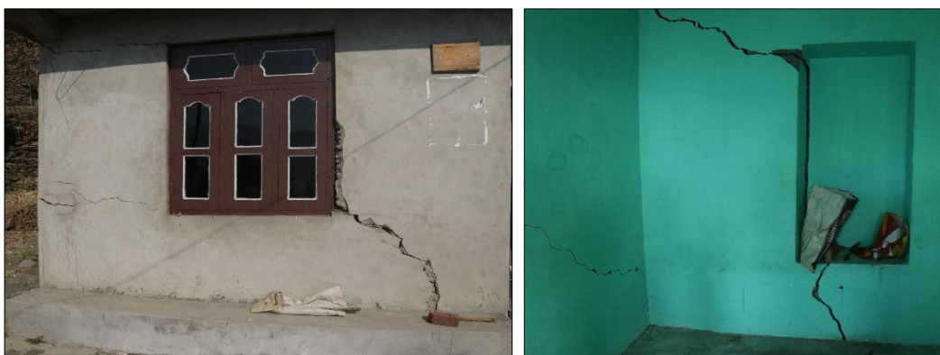
Large cracks developed on walls of houses.
