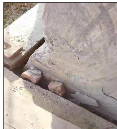
Displacement of building under construction.
