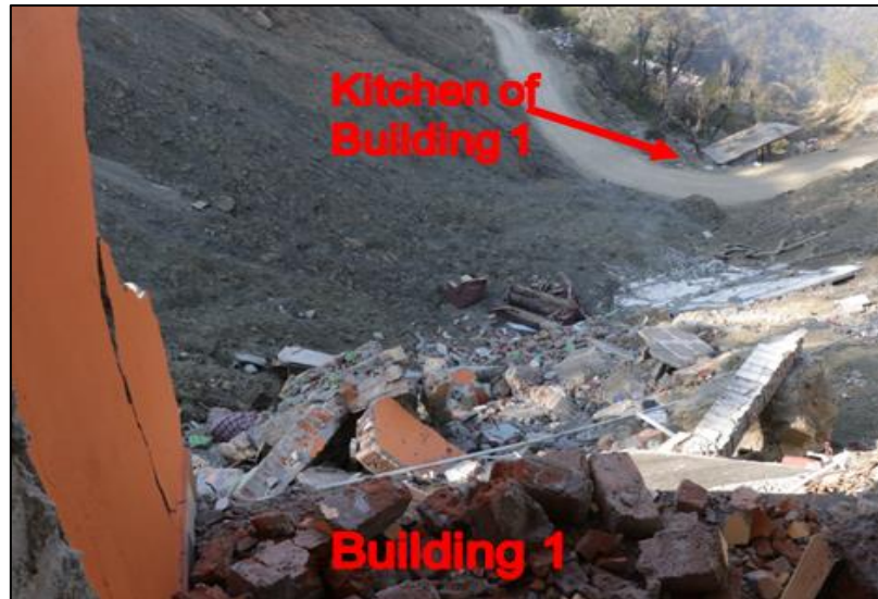
Displaced part (kitchen) of building 1.
