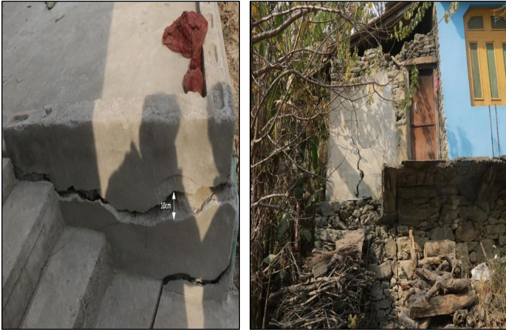
Cracks in residential buildings above landslide at site 1.
