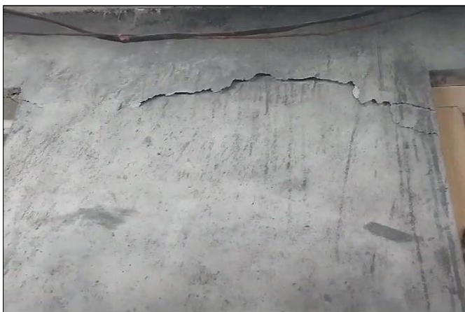
Cracks developed on the wall of building under construction.
