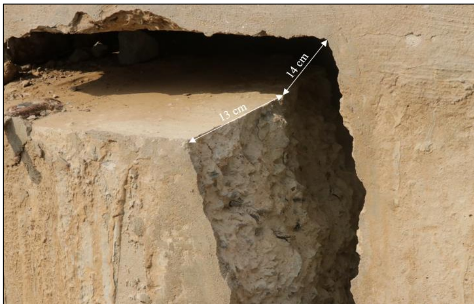
Cracks in retaining wall.
