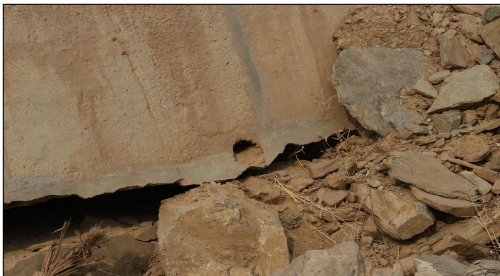
Clogging of weep holes.
