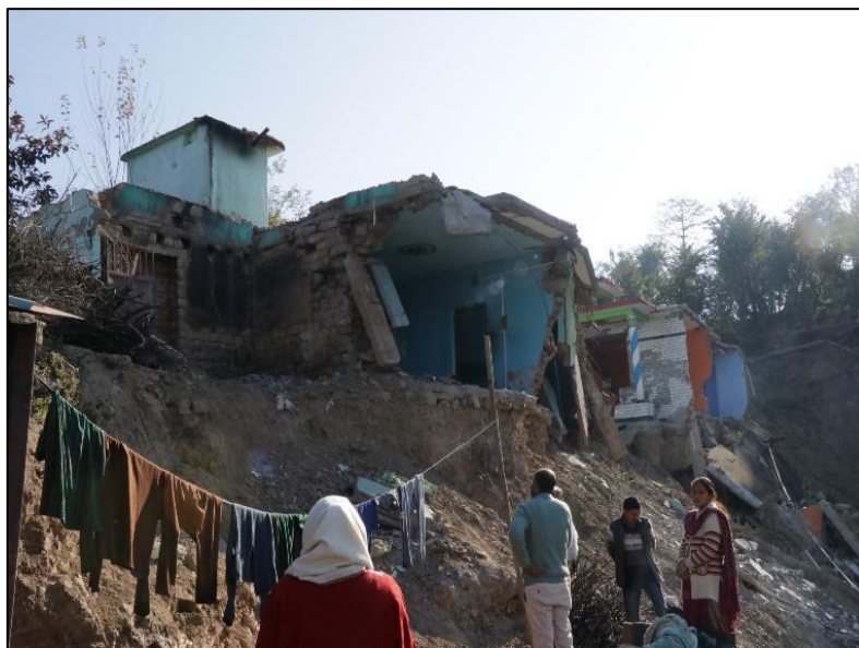
Complete failure of house.
