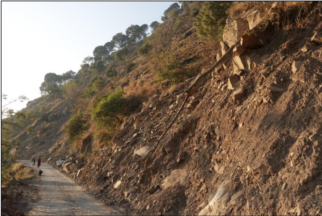
Landslide site above road.
