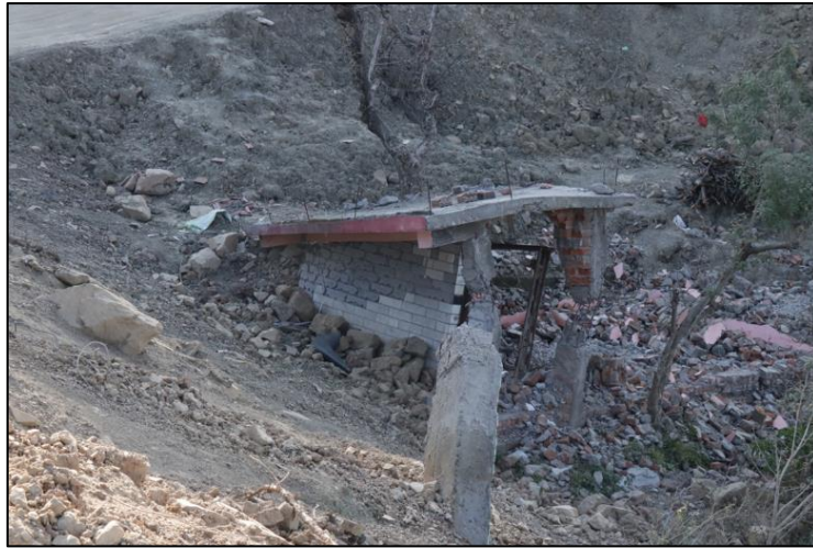
Fully damaged house.
