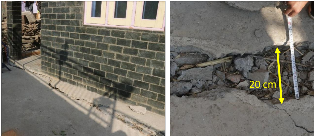
Cracks developed in houses.
