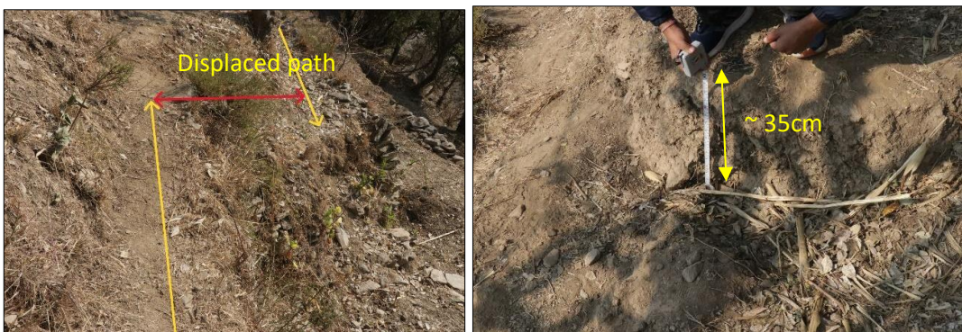
Road displacement due to settlement.
