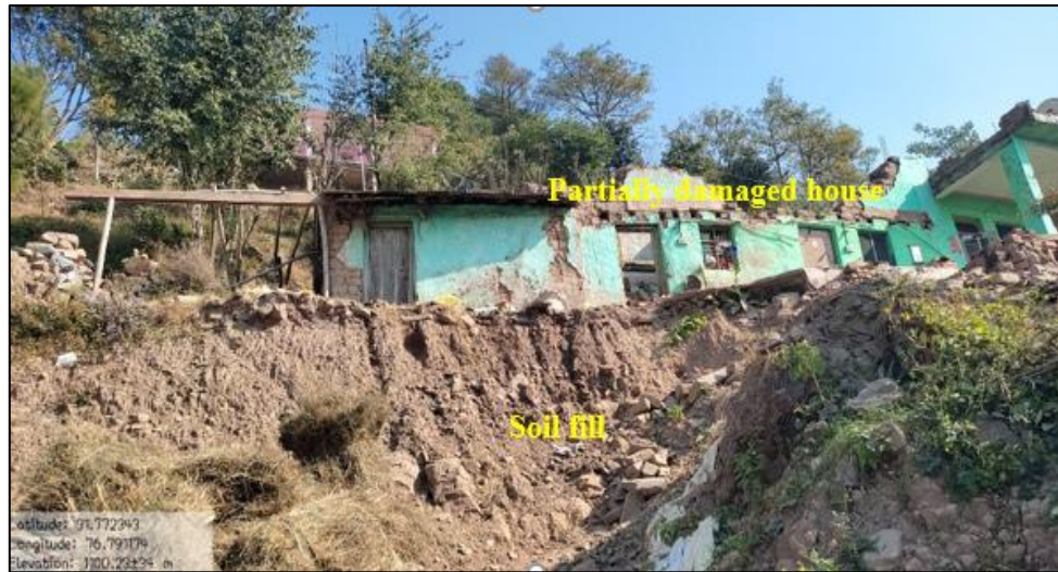
Partially damaged house.
