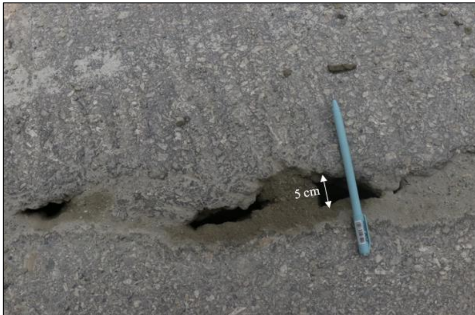
Cracks are seen on the road at the site.
