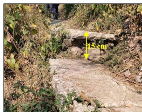
Settlement observed at site.
