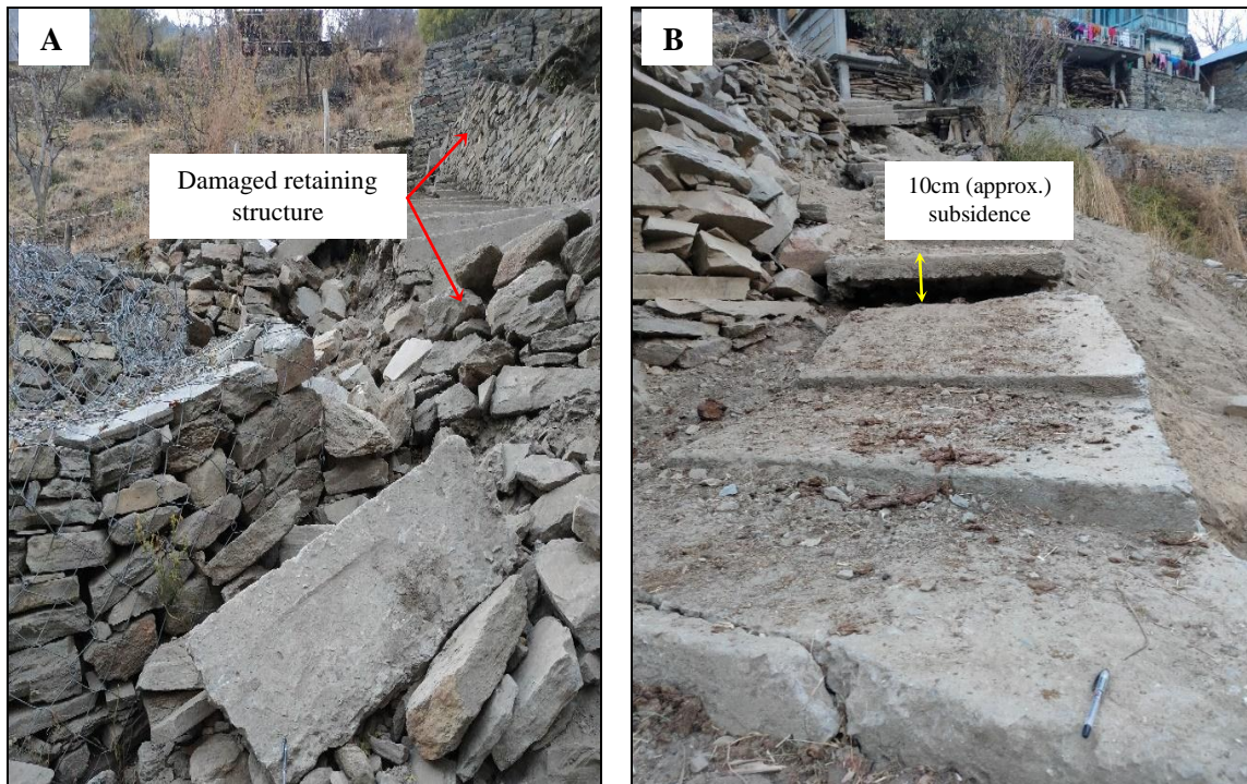
Fig. 13 Landslide induced damages to the existing Gabion wall (A) and a concrete stair pathway (B)
