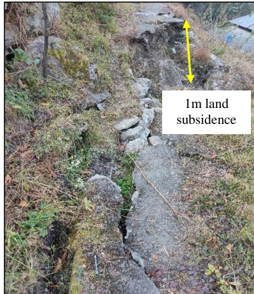
Fig. 24 Footpath damaged due to land subsidence
