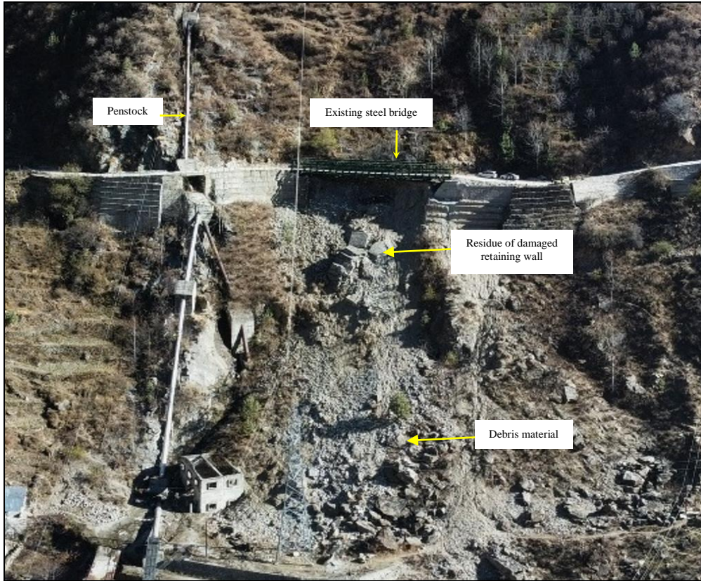
Fig. 27 Field photograph of Yangpa-I landslide, Kinnaur, HP
