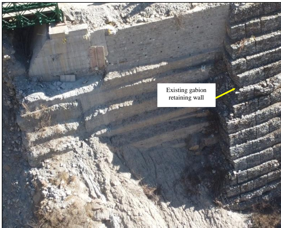
Fig. 28 Existing retaining structure at risk due to landslide occurrence
