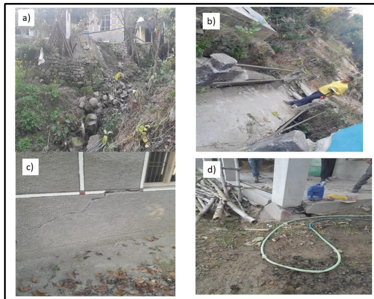
Fig. 29. Shows damage cause in the middle part of the slide zone to housing and erosion of the retaining walls along the natural drainage b) damage of cemented path c) development of cracks in building d) displacement of pillar and damage caused.
