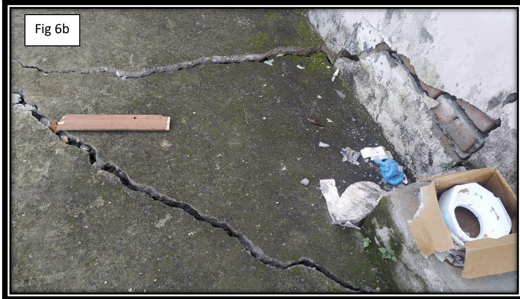
Fig 6 (a) and 6 (b) showing damages caused to the houses during the landslide incident in Parmar region. The development of cracks in the walls and floor indicated subsidence cracks.
