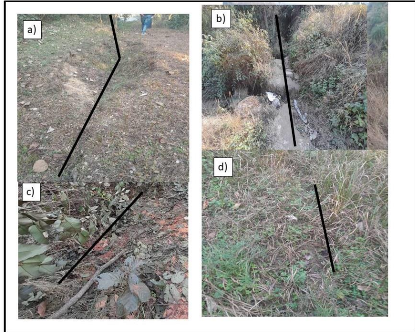
Fig.28 a, c ) Shows the development of land fissure and its direction at the summit of the landslide zone Images b) indicated the natural drainage present in the same summit zone by running along the slope direction. d) Again showing the direction of the fissure developed in the upper part of the slide zone.
