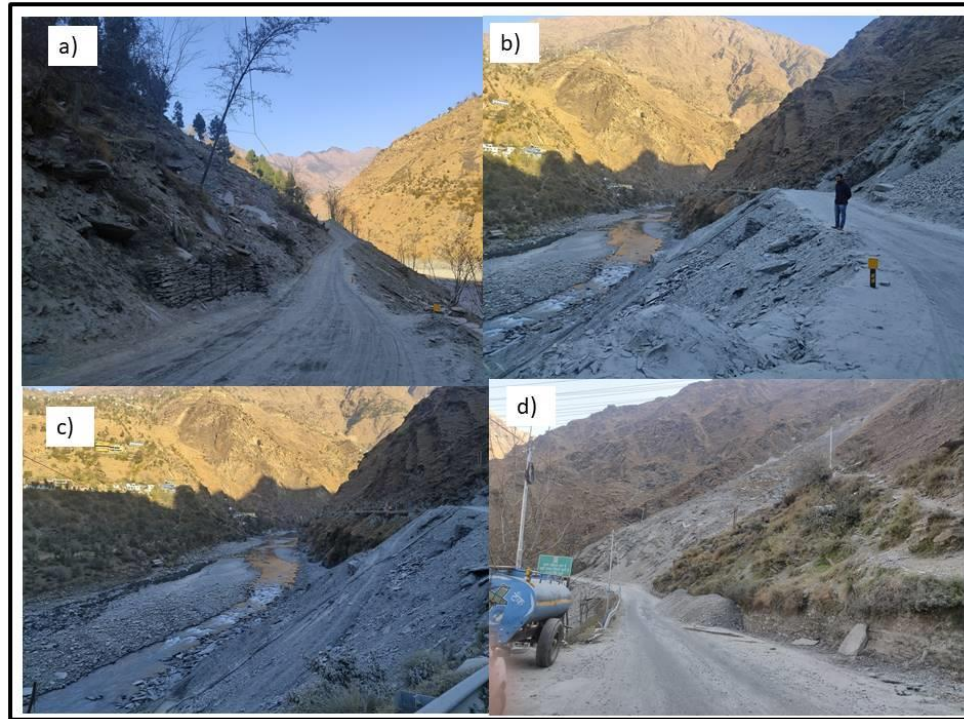
Fig.43: Lothal slide zone where presence of shear zone slope angle and water scoring action leads to toe erosion and further movement of the hill slopes and cause damage to the road.
