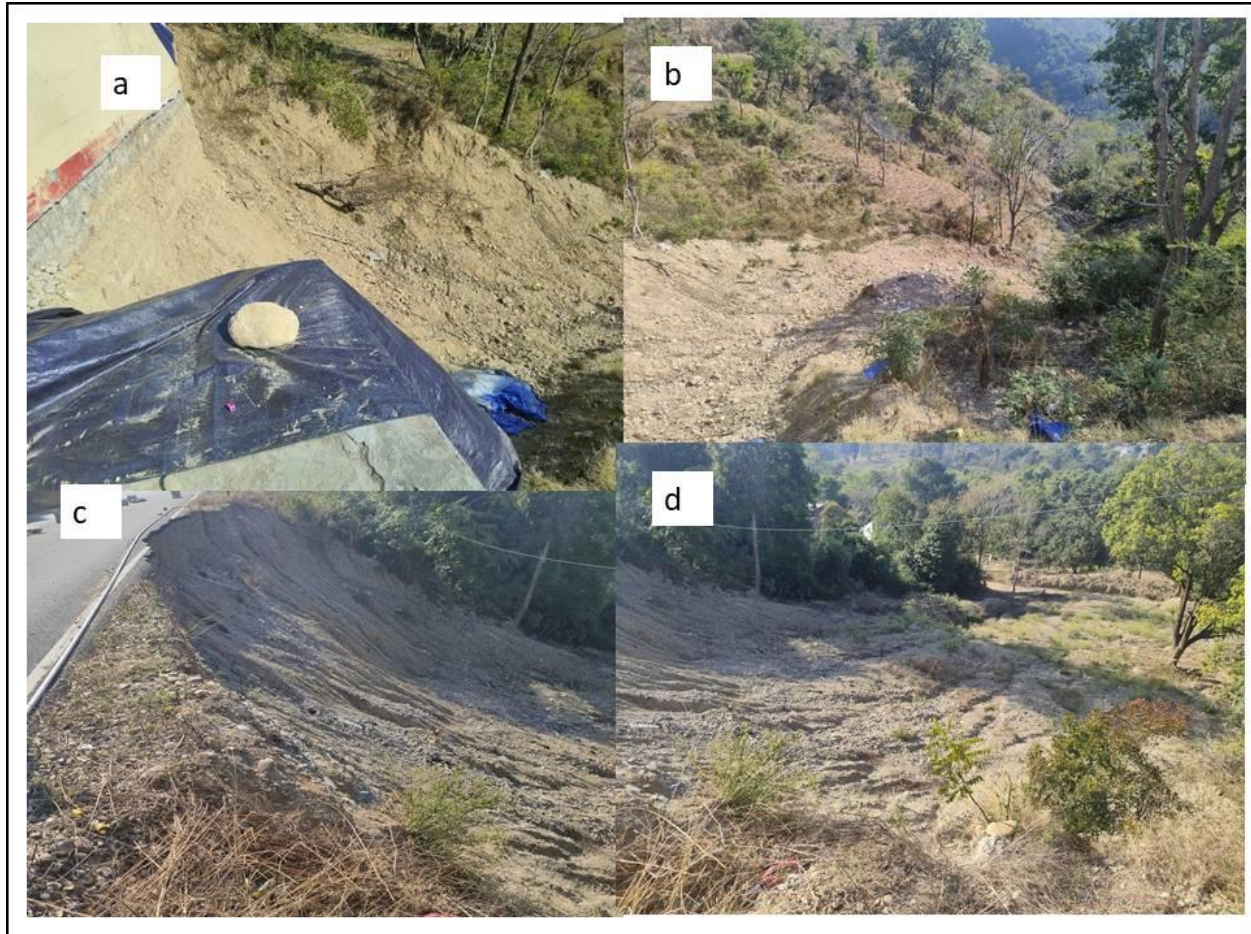
Fig. 11 Shows the lithology of the slide zone, characterized by gravelly soil, is evident in the displacement of the retaining wall observed on the upper right-hand side, which occurred due to the combination of heavy load and rainfall on August 14, 2023. The upper left photo illustrates the slope angle and pattern, while the lower picture depicts a slide along the National Highway in the same village, just a few meters downstream. Once more, the inability of the lithology to withstand the high moisture content in the gravelly soil resulted in a loss of frictional strength, leading to downslope.
