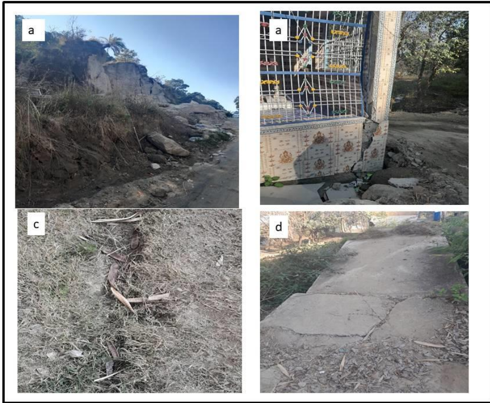
Fig. 23 Images showing hillock of the Middle Siwalik rock behind which the water was logged during heavy rain fall b) showing the damage caused to the temple due to subsurface movement. Land fissure developed in agricultural land downstream d) damage of cemented path leading to houses.
