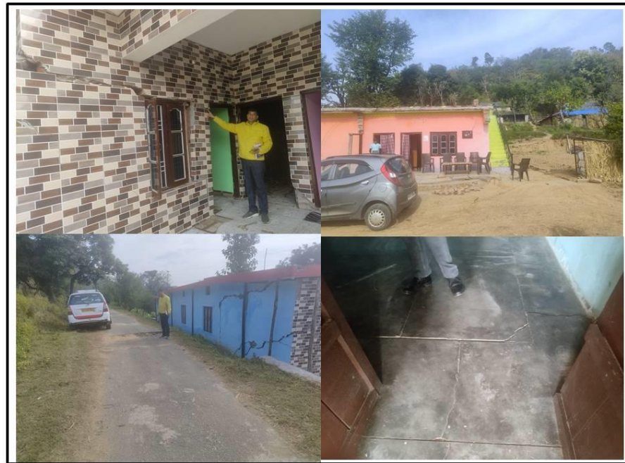
Fig. 21 Shows development of cracks in the tiles and displacement of walls b) the frontal part of the houses was totally damaged and the existing one developed wide cracks in the wall indicating subsidence cracks c) Again diagonal cracks in the walls and D) floors indicating subsidence features.
