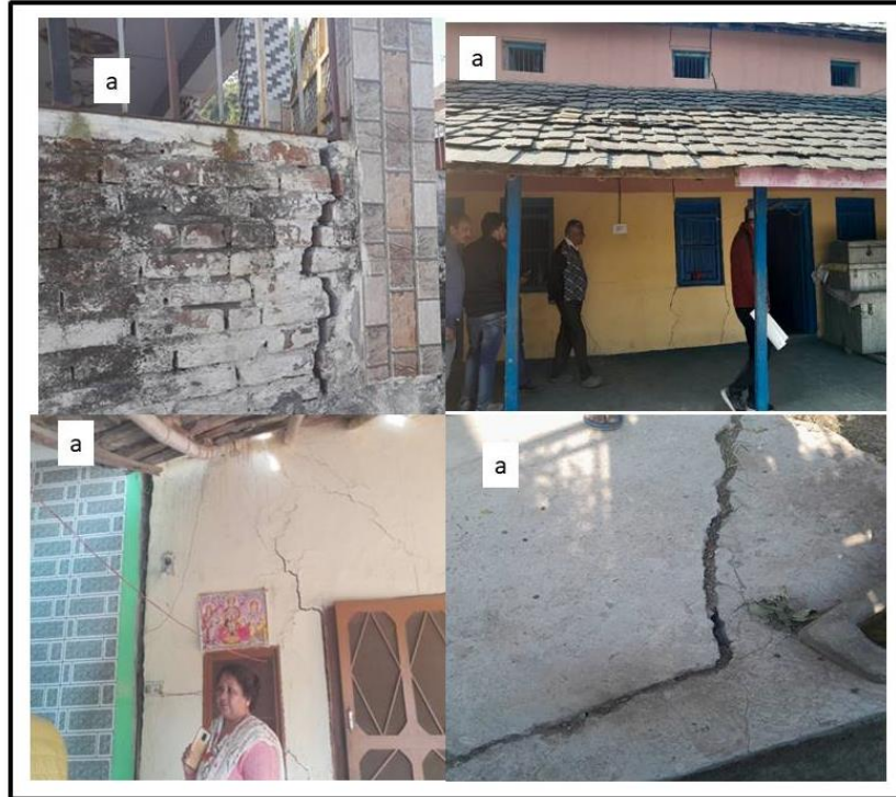
Fig.26. Shows subsidence crack in walls, and roads due to water logging and poor drainage system in the village. No doubt high intensity rainfall contributed to the damage but the moisture already present in the soil got accelerated by high intensity rainfall and thus developed subsidence crack at Pokhru village.
