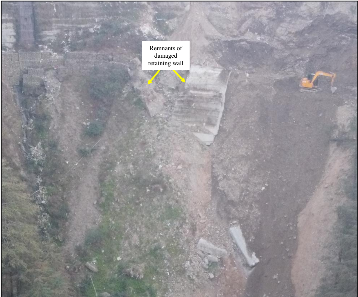
Fig. 53. Vegetal cover loss and damp underground conditions
