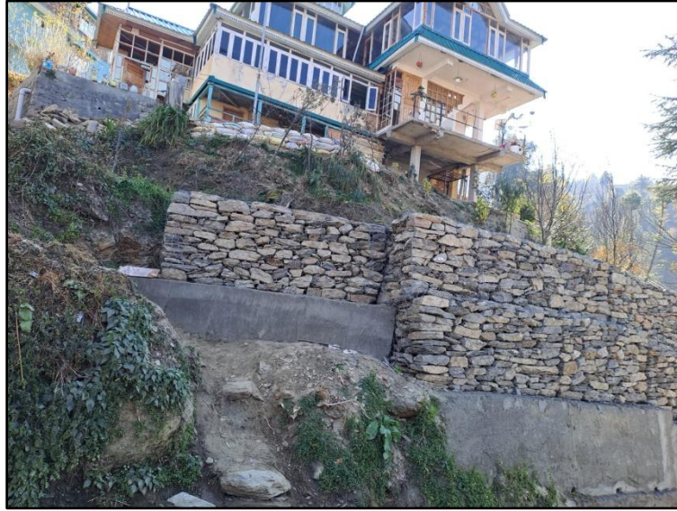
Fig. 44. Protection wall erected to support upslope structures and mitigate landslide impact
