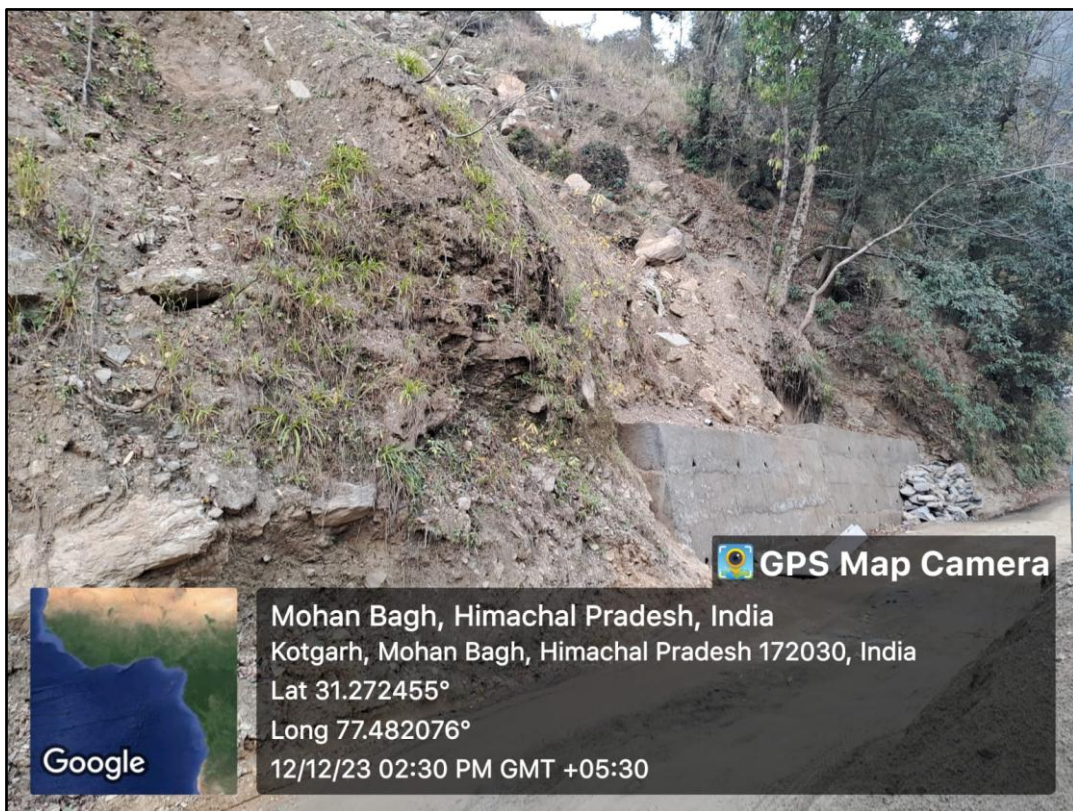
Fig. 57. Debris runout and protective measure
