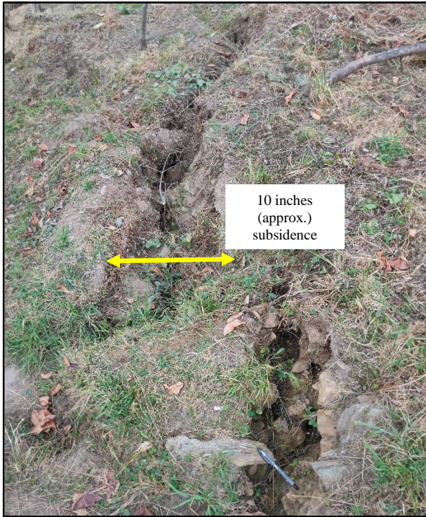
Fig. 58. Cracks as a risk for future land subsidence
