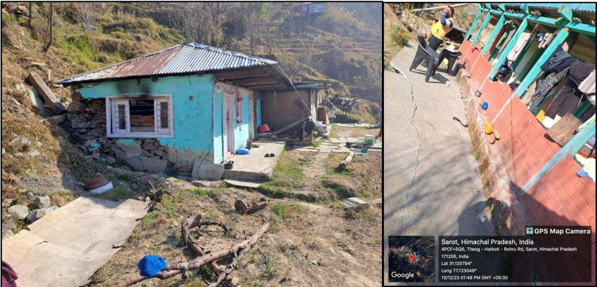
Fig. 37. Houses Affected by Land Subsidence in Plotidhar
