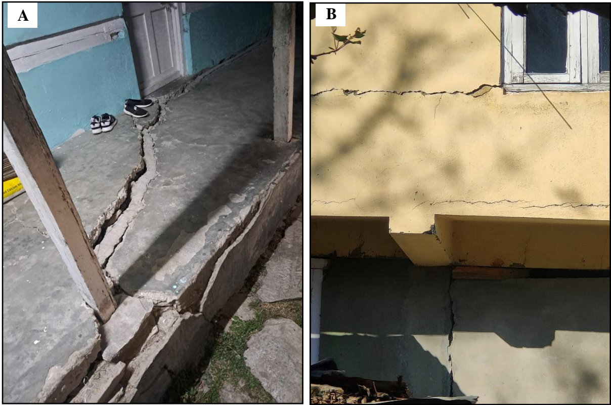
Fig. 67. Evident tension cracks in residential structures indicating subsidence
