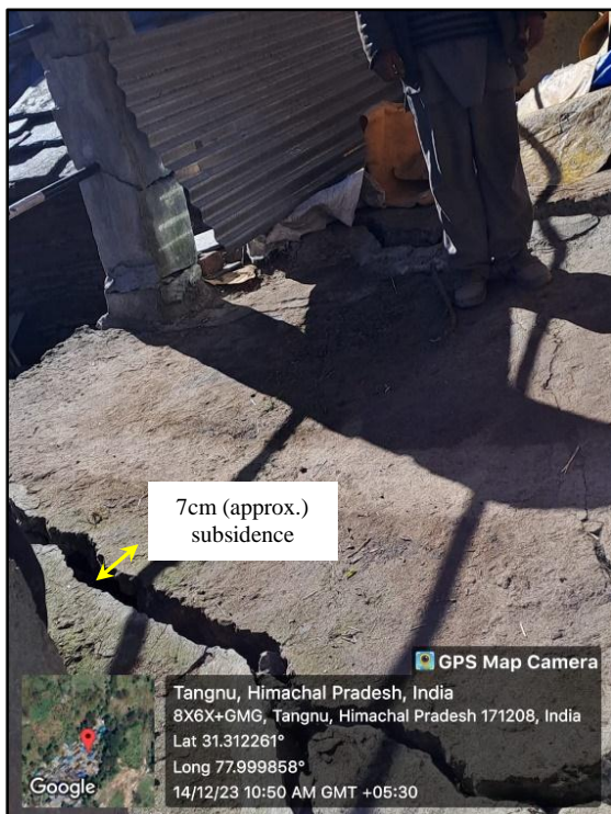
Fig. 18 Cracks in Houses
