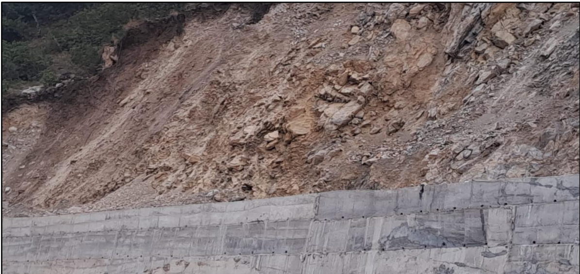
Fig. 12 Disintegrated rock mass and mitigating concrete retaining wall
