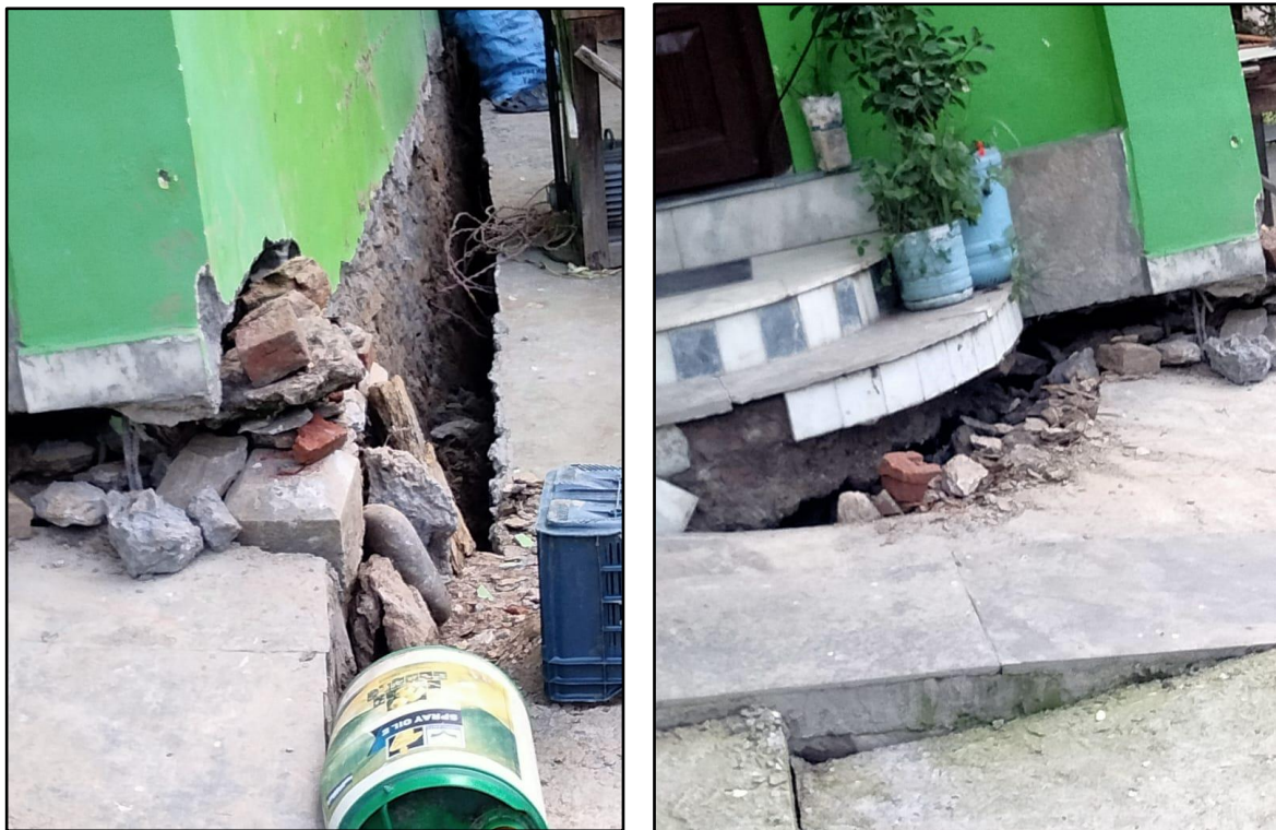
Fig. 43. Structural damage from land subsidence
