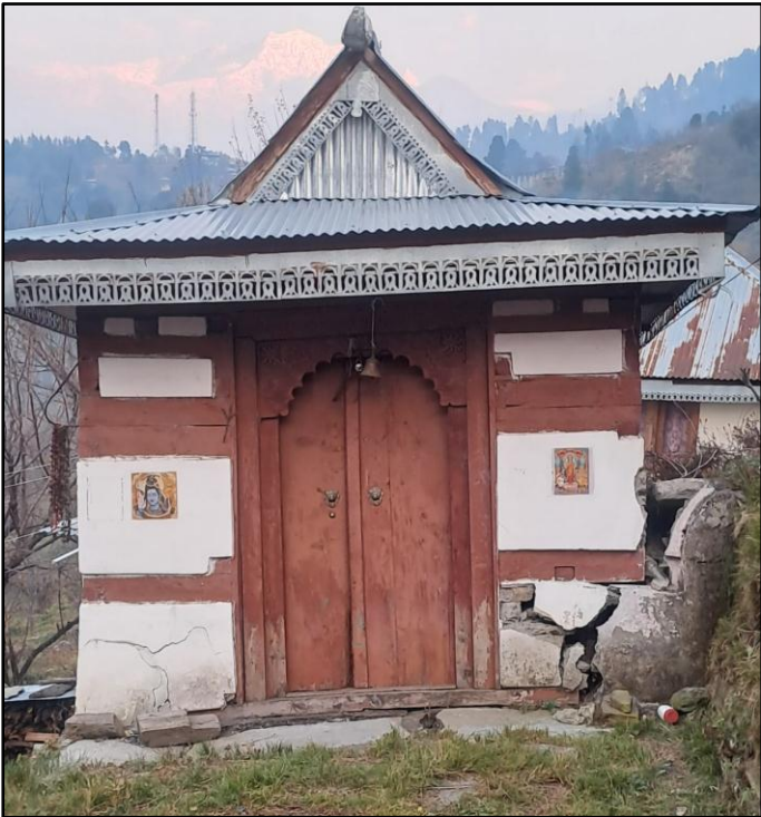
Fig. 68. Temple affected due to subsidence
