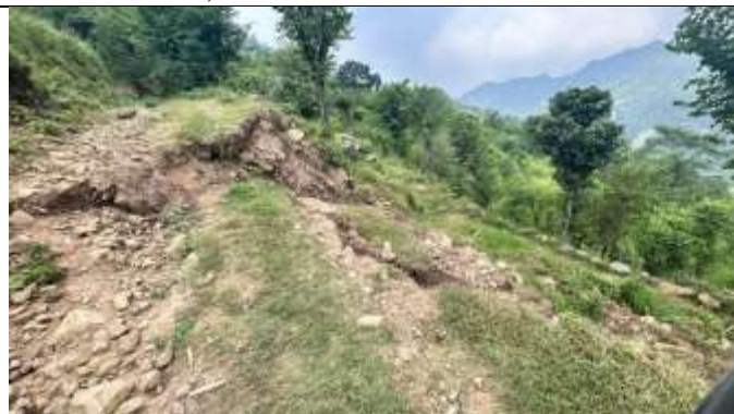
Figure 10 (v) Land Subsidence and tension cracks observed near Badhiyar village
