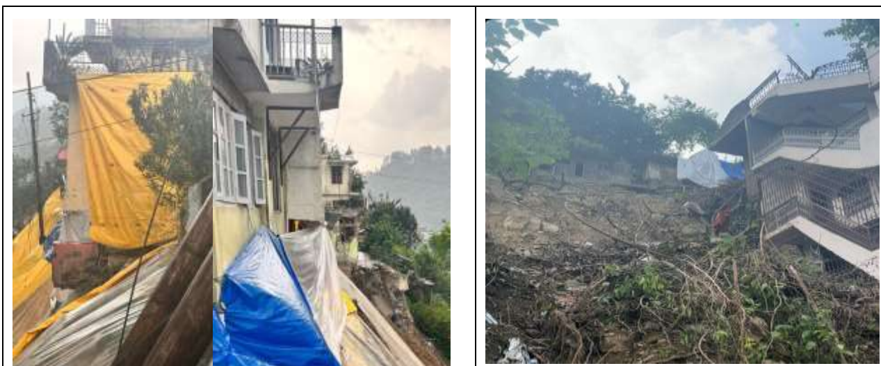
Figure 5 (d) Showing unscientifically constructed civil structures over unconsolidated material.
