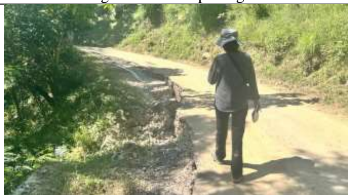
Figure 10 (n) Observance of ground craks on raod near Chanauta Village
