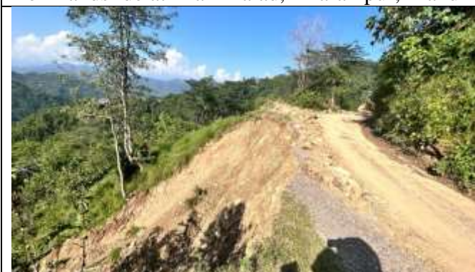
Figure 10 (i) Caving of road due to landslide at Banal village
