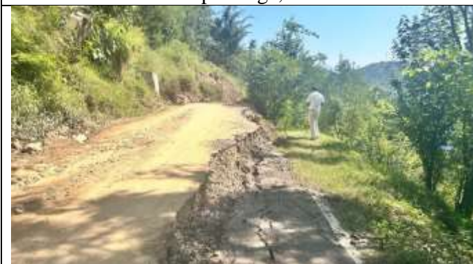
Figure 10 (m) Subsidence observed near road at Brahmfalad village
