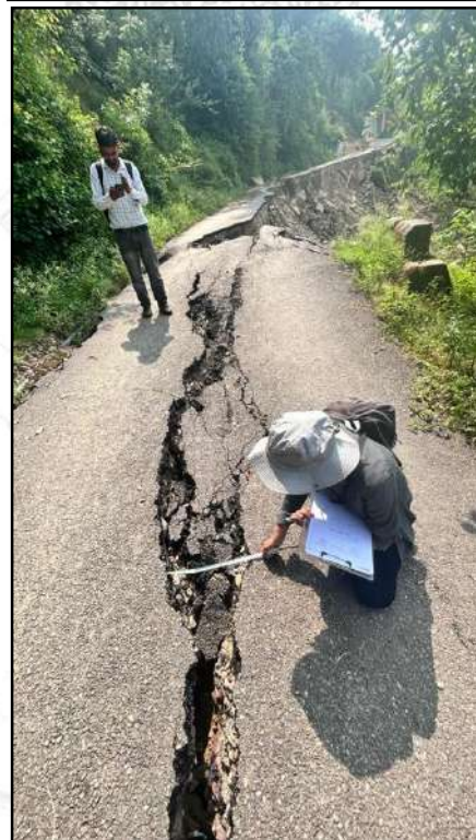
Fig: Road damaged and subsided
