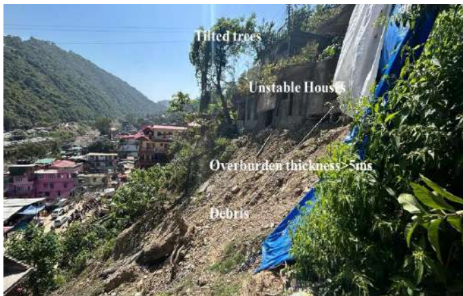
Figure 4.6 Steep slope exposing loose debris material at crown
