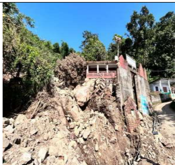
Figure 7(b) II. Damaged Govt. School, Juccain, Sarkaghat, Mandi premises
