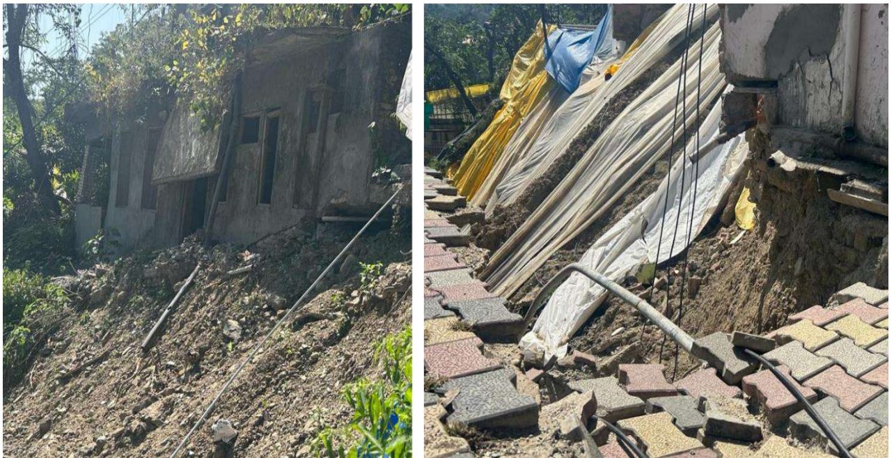
Figure 4.21 Unscientifically constructed houses posing a major threat during natural hazard
