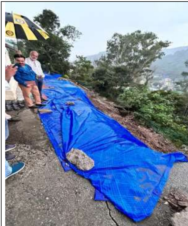
Figure 6 (f) Debris Slide at Judge House, Mandi with tension cracks covered by plastic sheets to avoid further percolation of water
