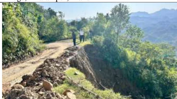
Figure 10 (j) Caving of road due to landslide at Banal village
