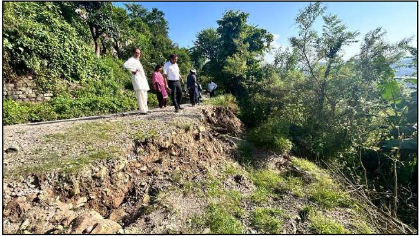
Fig 2: Road subsidence ( \pm 2.5 feet)
