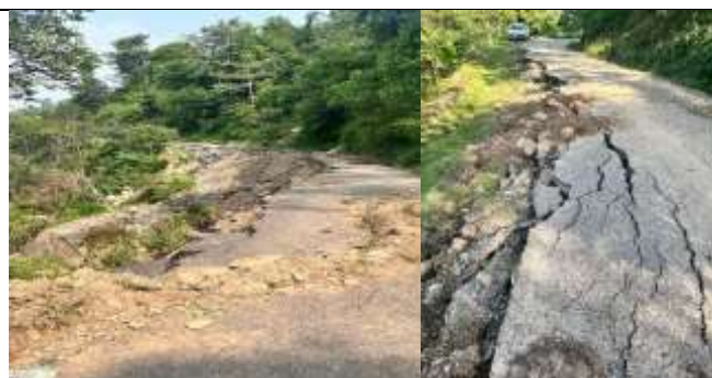
Figure 10 (h) Ground cracks on roads of Badhiyar village, Dharampur, Mandi
