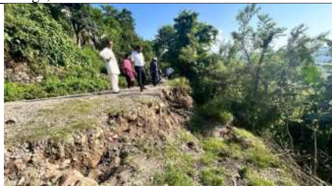
Figure 10 (q) Subsidence of land >1m on road near Brahamfalad village, Mandi
