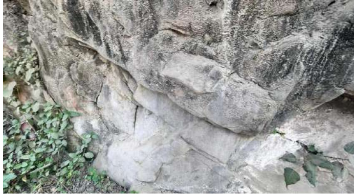
Figure 4.20 Joints having clay to calcitic filling in joints
