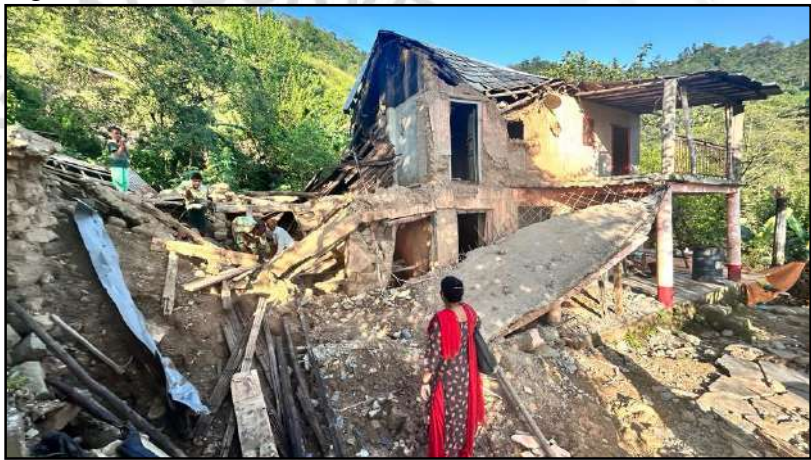
Fig 3: House damaged by slide.
