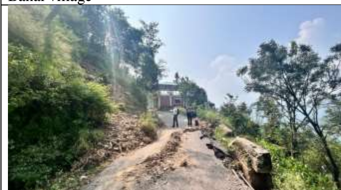
Figure 10 (k) Ground cracks observed on road due to landslide at Mandap village, Mandi
