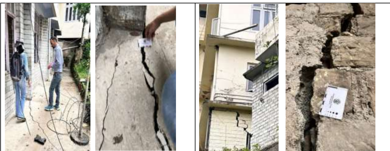
Figure 6 (h) showing wide ground cracks observed in the IPH building
