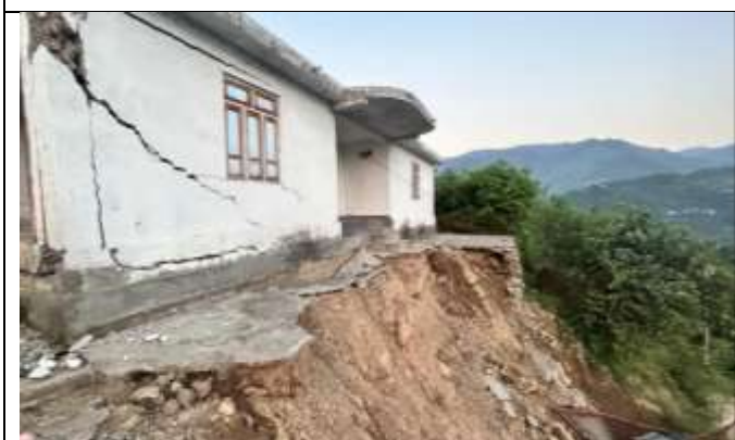
Figure 10 (y) Damaged houses due to slide at Didnu Village
