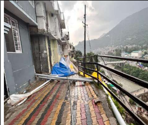
Figure 4.1 Slide leading to collapsed pathway, damaged the drainage pipes and channels during slide
