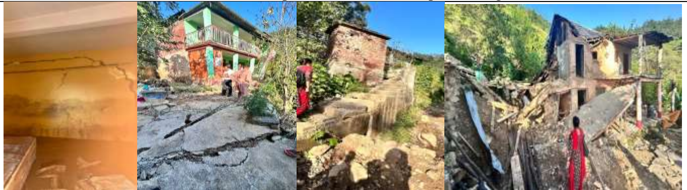
Figure 10 (d) Cracks observed on walls and floors of buildings and displacement of stairway due to landslide near Riyur and Collapsed building near Riyur village, Mandi district, HP
