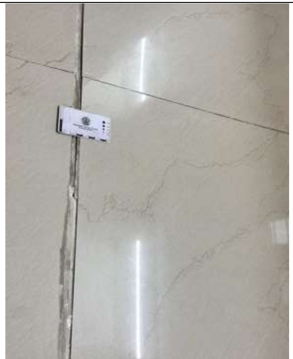
Figure 6 (g) Cracks on floor of house repaired by filling by cement/ other cementing materials
