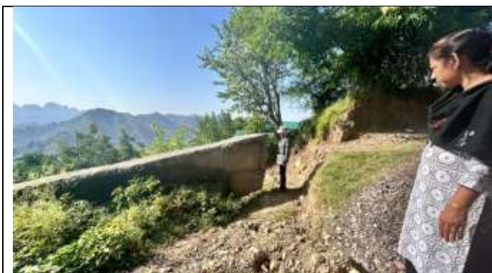
Figure 10 (o) Subsidence of land >5m near Banal village, Mandi district. HP
