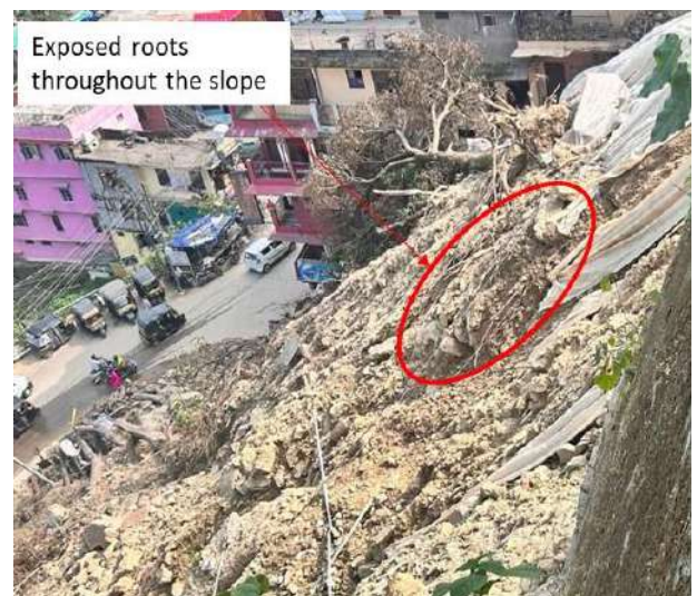
Figure 4.16 Exposed roots throughout the distressed slope
