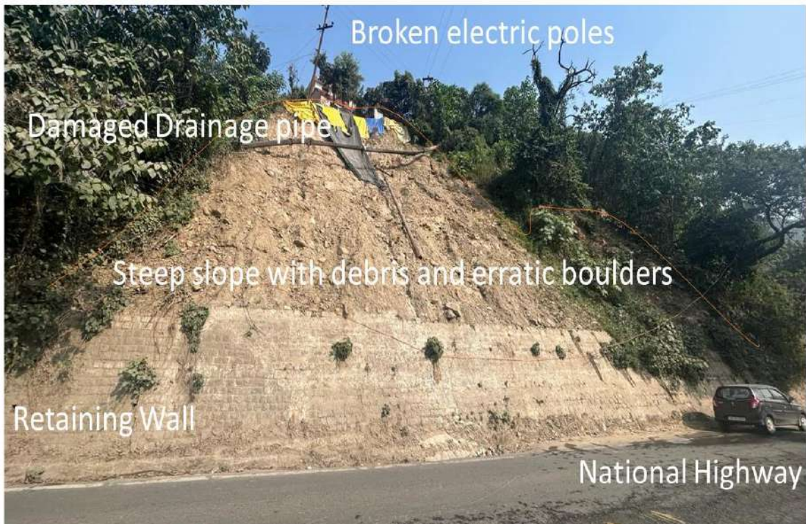
Figure 5.2 The active scarp characterized by steep slope exposing loose debris material
