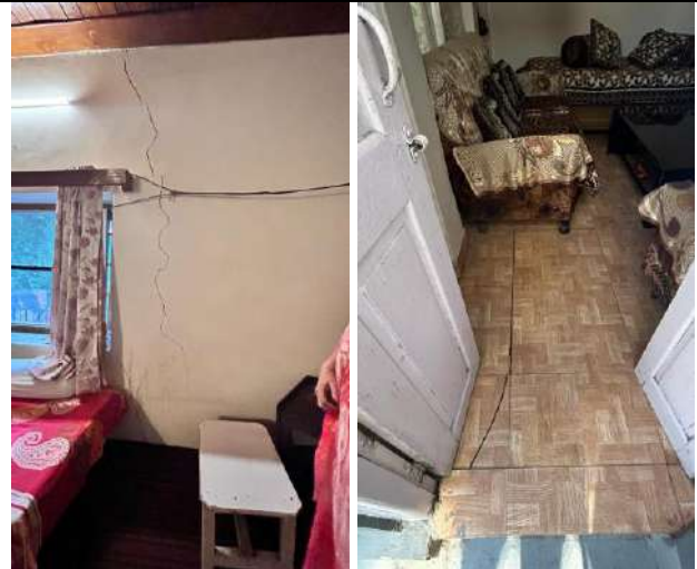
Figure 4.2 Diagonal cracks observed on the walls and floors of houses
