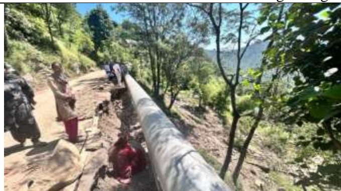
Figure 10 (u) Caving of road and development of tension cracks om roads near Barouti village
