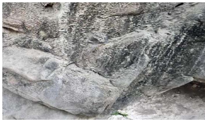
Figure 5.6 Joints having clay to calcite filling in joints
