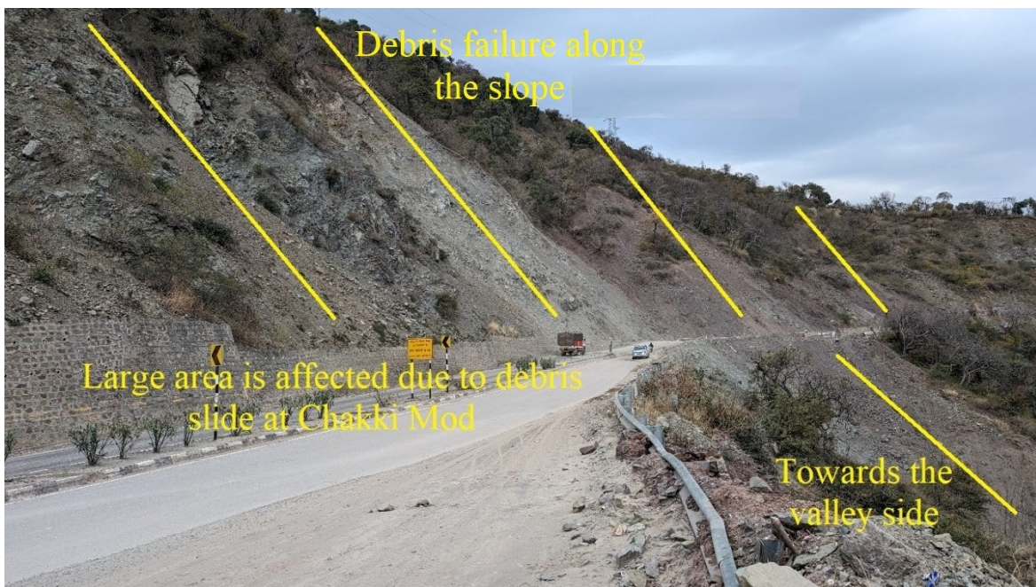
Fig. 8 - A panoramic view of debris slide at Chakki Mod.
