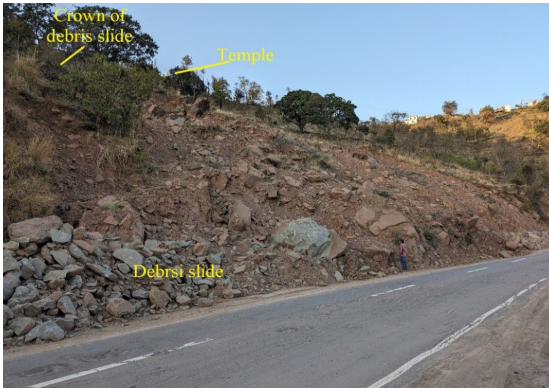
Fig. 10 The debris slide, the slide is also growing towards the upside (progressive slide).
