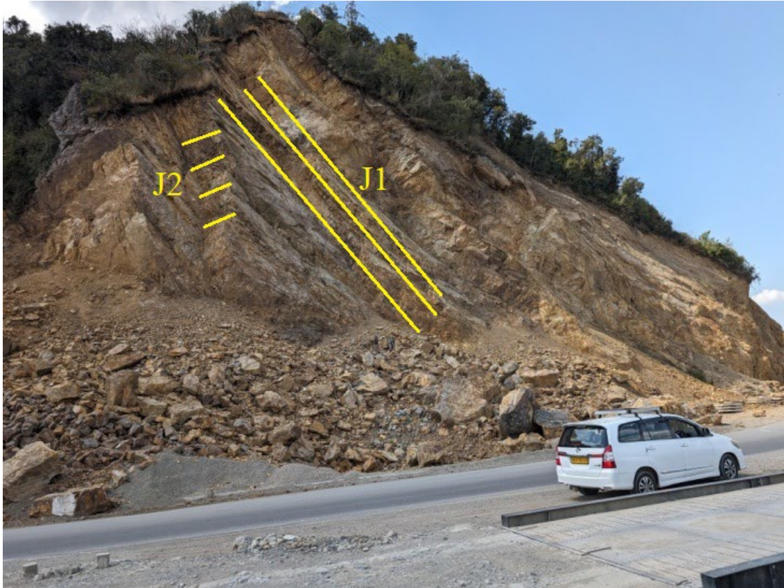
Fig. 1 Planar failure (due to joint J1) along the National Highway (NH-5) between Parwanoo and Kandaghat in Solan district. Yellow lines show joint sets.
