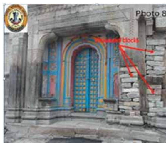
Damage on the Eastern side of the Temple from where the water rushed in
