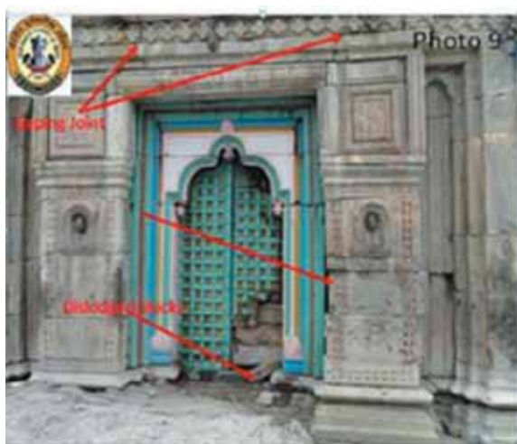
Damage on the western gate of the temple from where water gushed out
