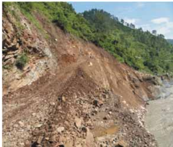
Slide in RBM at Naulapani (Tilwara-Rudraprayag)
