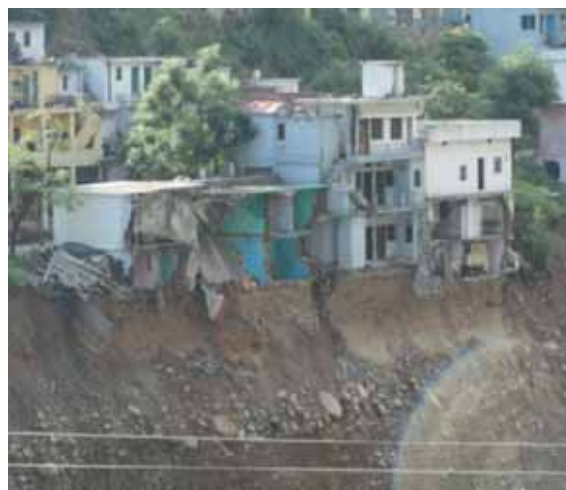
Damaged to civil structure in Sumari area
