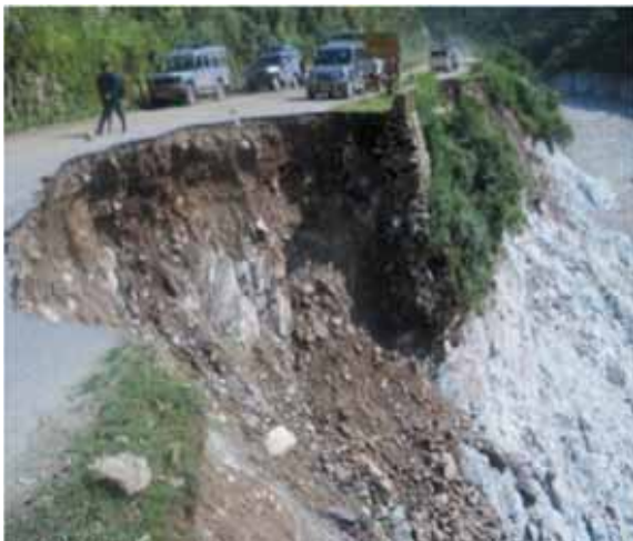
Road Breach in RBM Near Naulapani (Tilwara-Rudraprayag)
