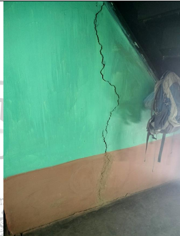
Fig. 11: Horizontal and vertical cracks observed in a house with mud plastering.
