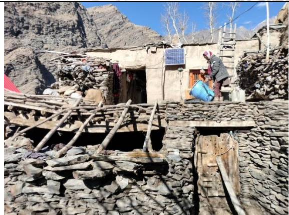
Fig. 12: 80 year old highly damaged mud house built on rock piles with no proper foundation.
