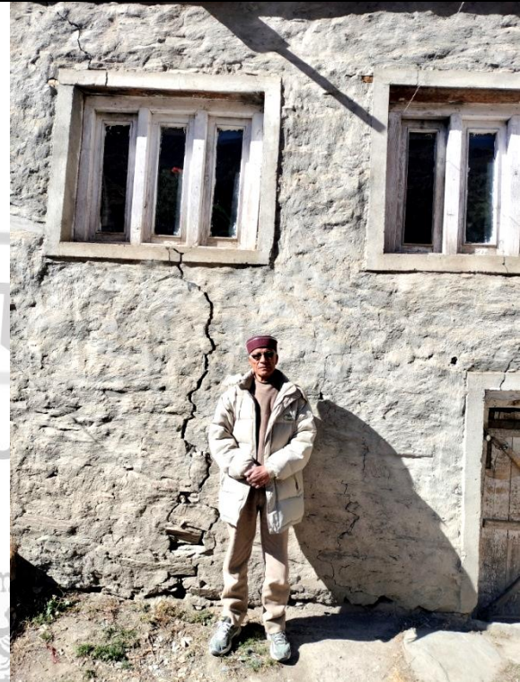
Fig. 15: Vertical cracks seen cutting across the wall along with the wooden window frame.
