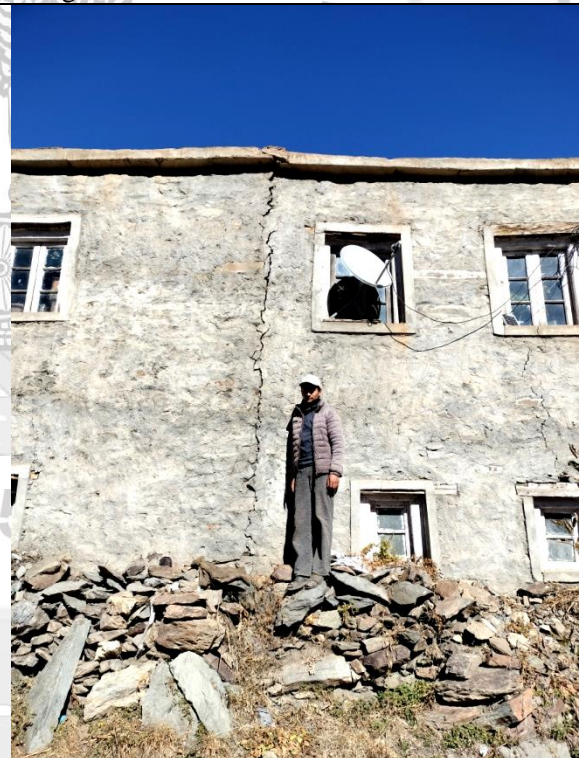
Fig. 17: Subsidence near the house has led to the formation of irregular vertical cracks.
