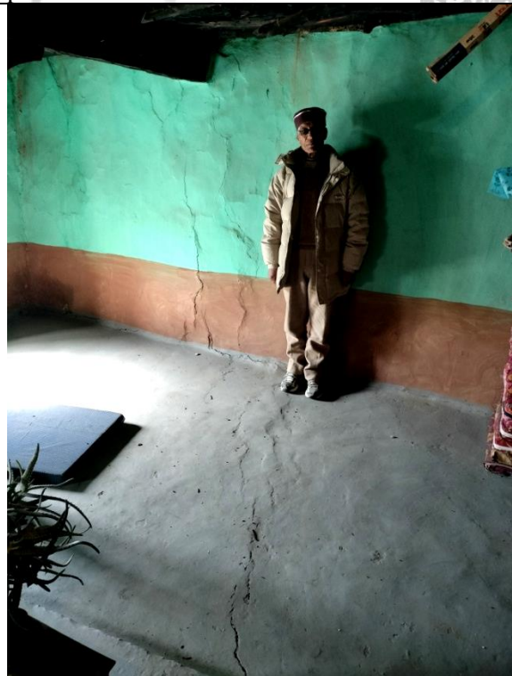
Fig. 16: Cracks on the floor of a mud house can be seen continuing towards the wall.
