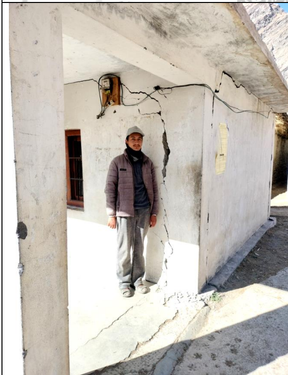
Fig. 20: Ground cracks continuing into the walls of a community centre. Note that the trend of cracks on the wall and ground is same.
