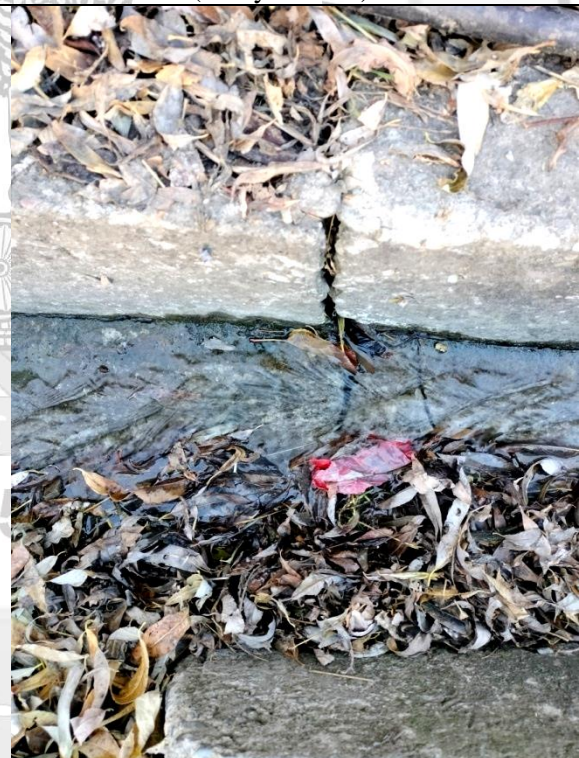
Fig. 21: Vertical cracks observed in a man-made channel with flowing water near a house leading to possible seepage of water to the ground.
