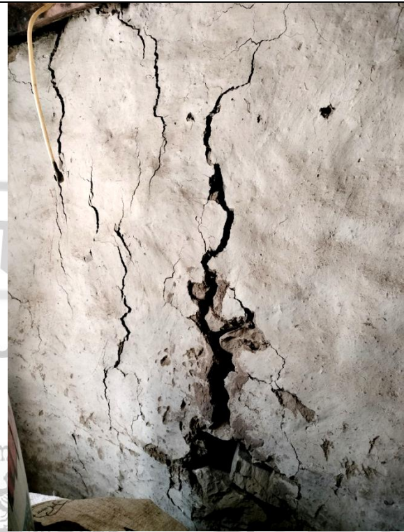
Fig. 19: Highly damaged and bulged wall of an old mud house (~80 years old).
