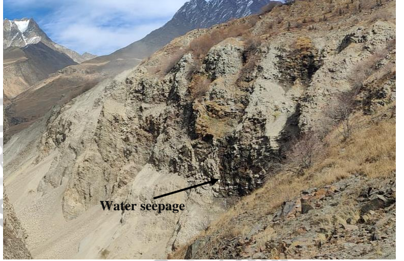
Fig.1: Distal view from right side of Lindoor Debris/Talus Slide 2, Lahaul & Spiti District with seepage of water.
