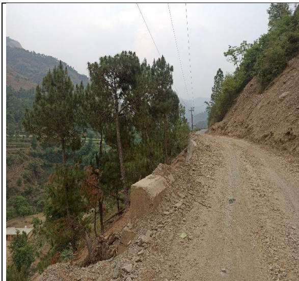
Fig. 3 State highway passing through slide zone & tree tilting indicating ground movement
