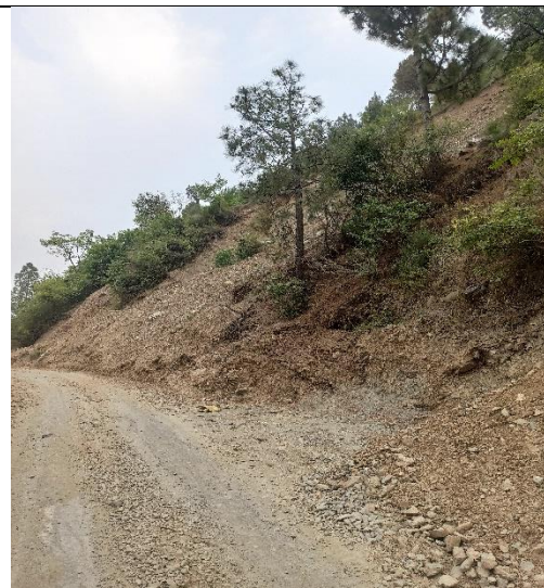
Fig. 4 Large debris overburden and minimum vegetation on hill side slope
