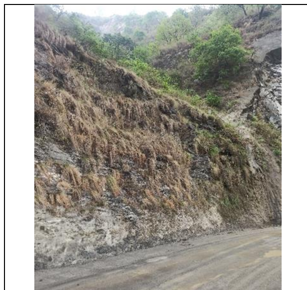
Fig. 1 Major water seepage at site
