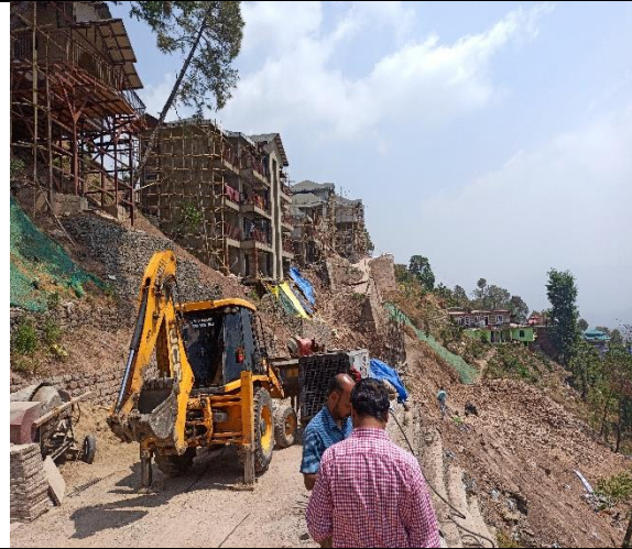
Fig. 2 Both hill and valley side instability and high building loads on slope
