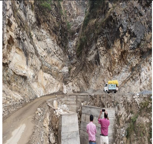
Fig. 2 Highly stresses jointed rock mass at site
