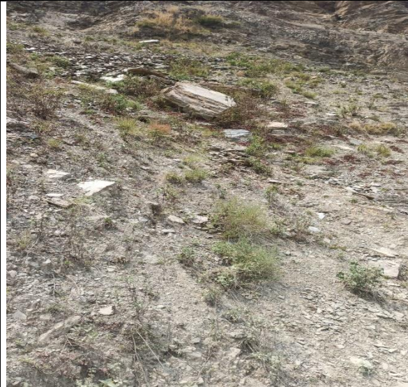
Fig. 4 Potential for rock fall and debris flow at site
