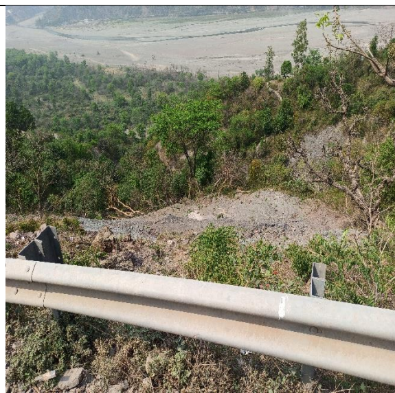
Fig. 2 Toe cutting by river below the slide
