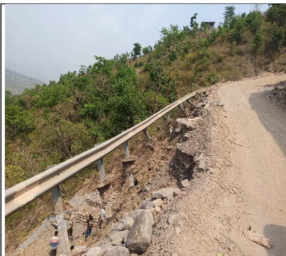
Fig. 3 Fine soil and debris material and erosion of road
