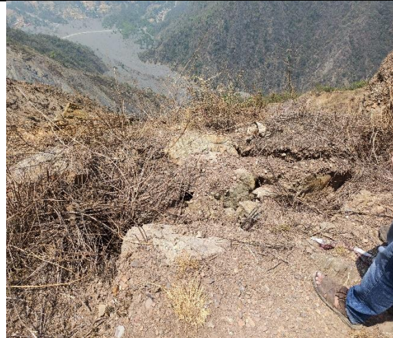
Fig. 3 Tension cracks observed on top of slide
