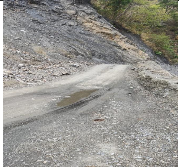
Fig. 2 Rock joint dipping towards road indicating instability
