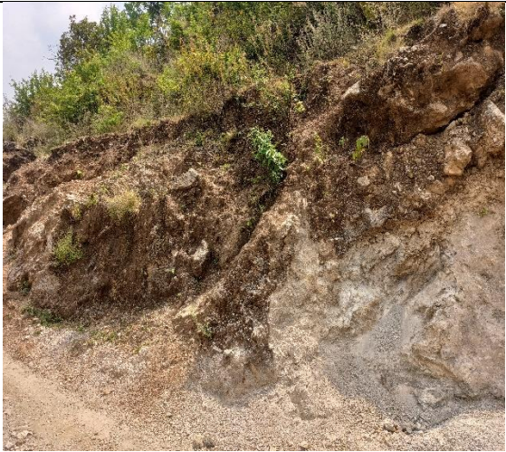
Fig. 3 Moisture present in strata indicating blocked drainage paths
