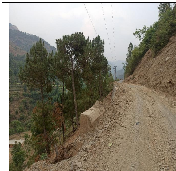
Fig. 1 Fine soil with debris material underlain by blocky rock mass
