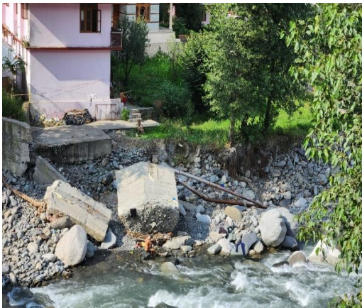
Figure 14 Foundation of The Structure Uprooted
