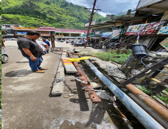
Figure 15. Dismantled poles After the Flood Impact
