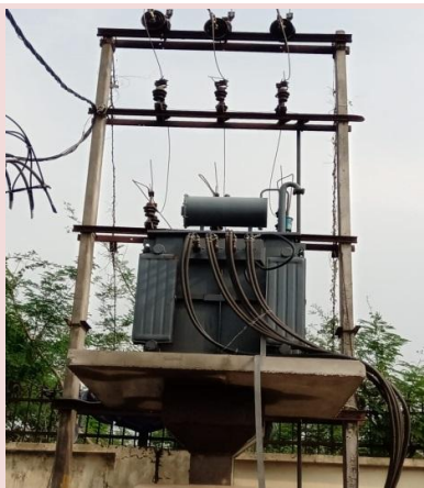
Figure 13 Plinth mounted prefabricated
