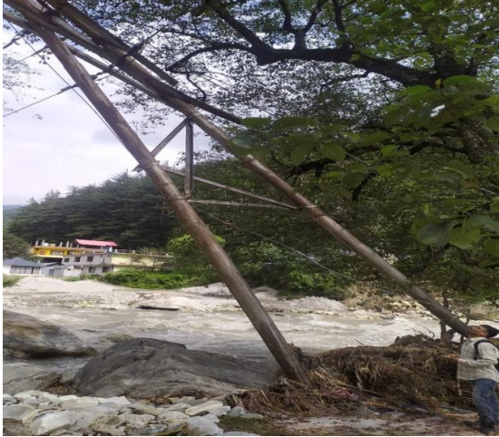
Figure 12 Deformed Poles Due to Flood
