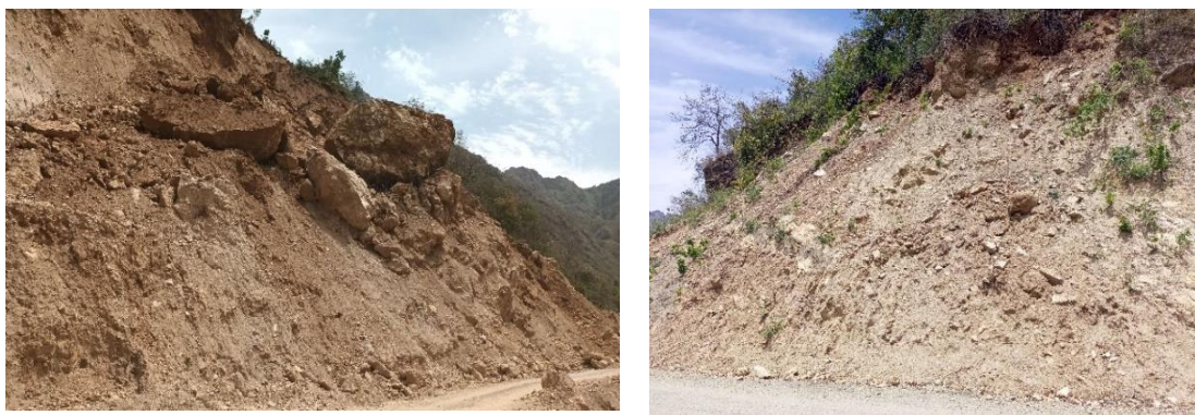
Figure 13: Landslides in Bilaspur district
