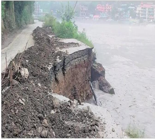
The Shimla-Mandi road near Tattapani experienced continuous sinking due to erosion by gushing Sutlej river water.
