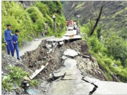
A road caves in following heavy rain in Chamba.
