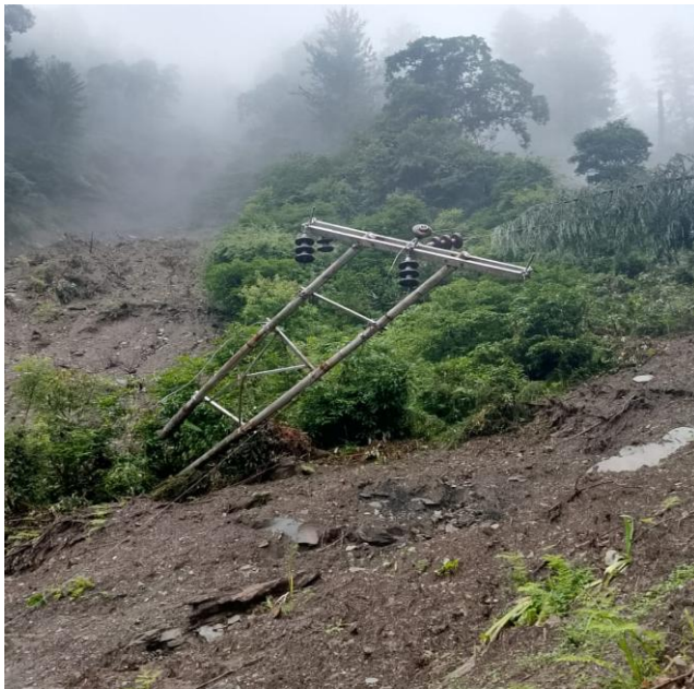
Figure 2 33 kV Thunag–Janjehli sub-transmission line
