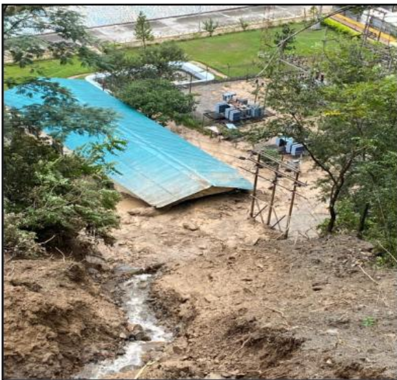
Figure 5 Showing Damage to Civil Infrastructure
