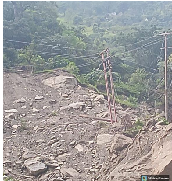
Figure 1 damage to the 33 kV Pandoh–Thalout sub-transmission line
