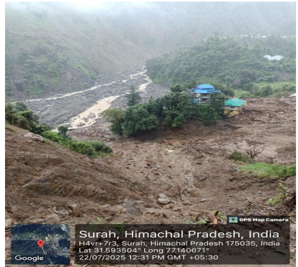
Figure 3 Washed-out site of 22 kV HT line at Surah
