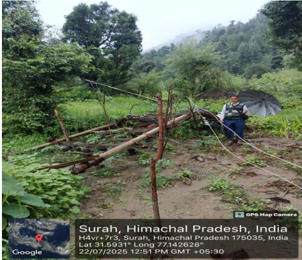
Figure 4 Damaged 22 kV HT and LT line
