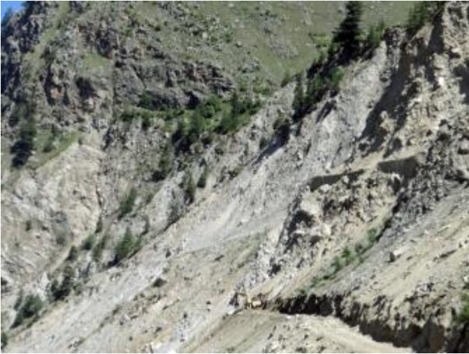
The damaged stretch of road near the Kuppa village in Sangla Valley.
