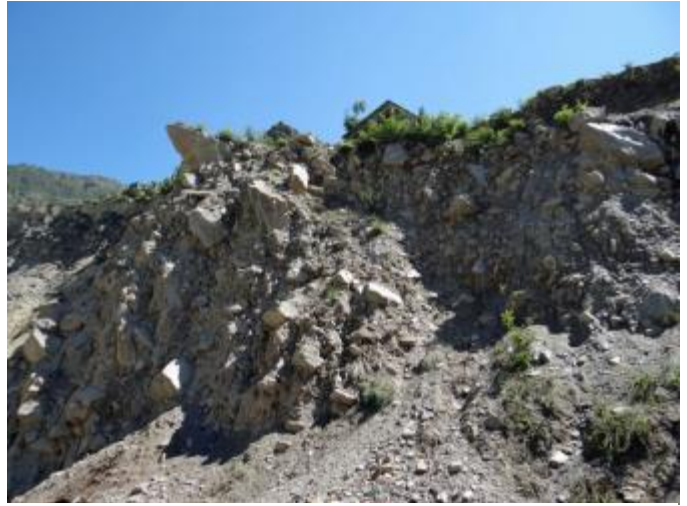
A house sitting on the top of a sliding slope.
