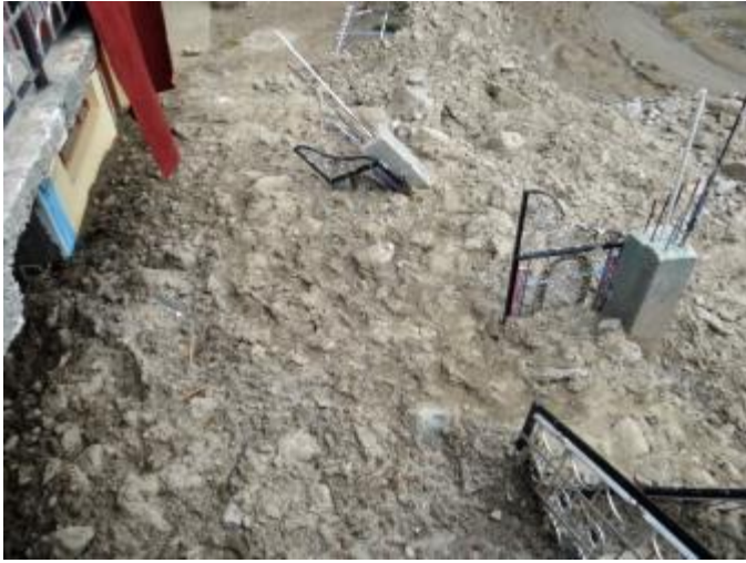
The destruction caused by the force of mud flow.
