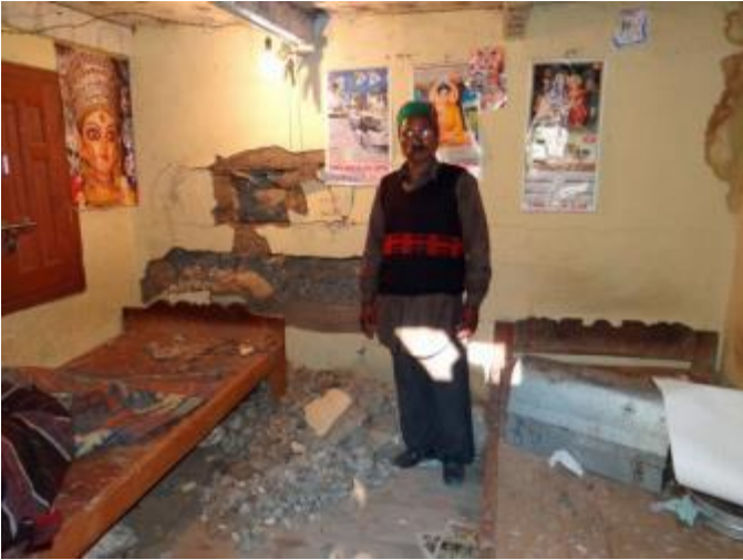
An inhabitant of Sangla village showing the damage caused to his house by a rock fallen during the landslide.
