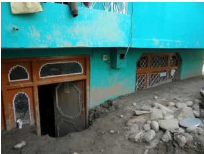
Mud flow covered the houses upto 5-6 feet.
