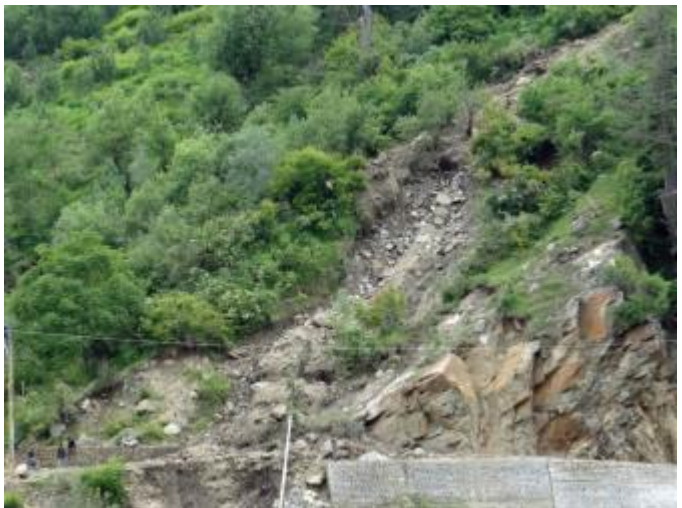
Local people assessing the damage caused by the landslide to a connecting road.
