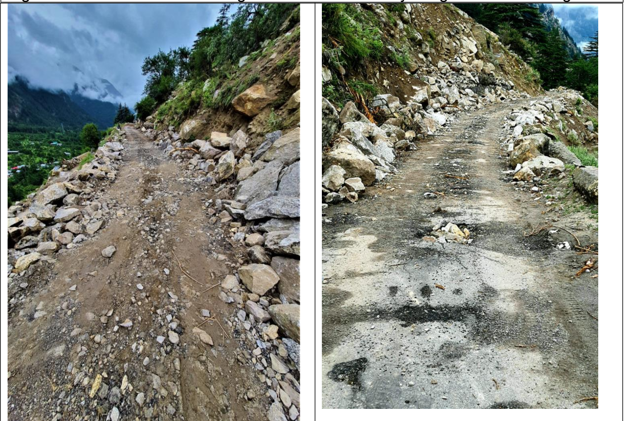
Fig.-11: Severely damaged Sangla- Chitkul road due to rock fall of 25th July 2021
