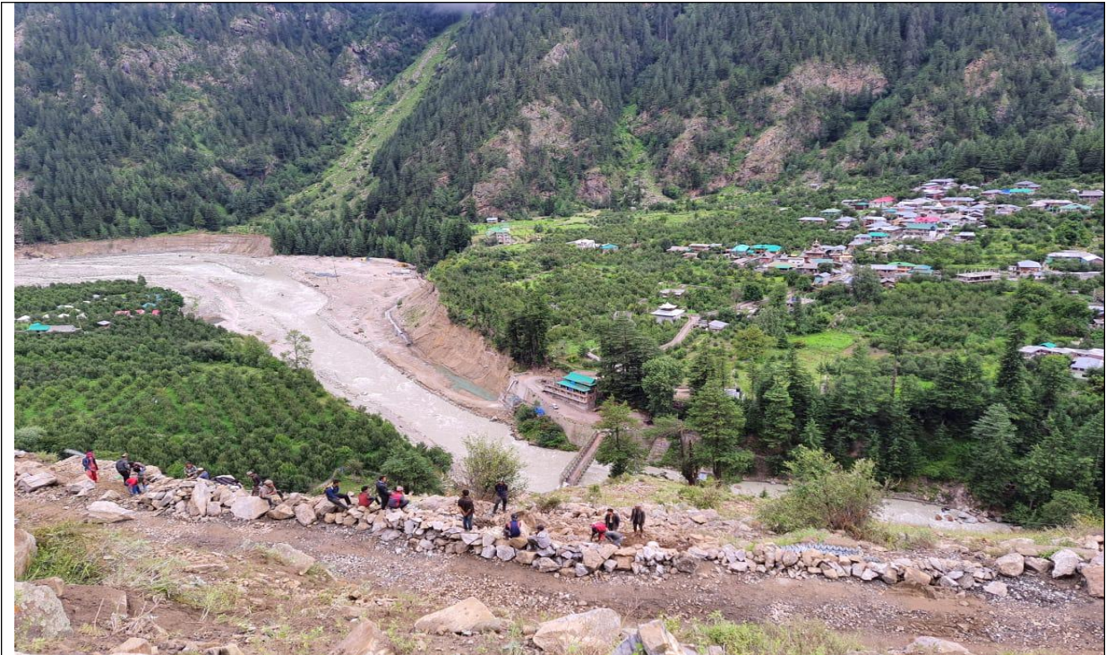
Fig.-10: Down hill view of damaged link road and bailey bridge to Batseri village
