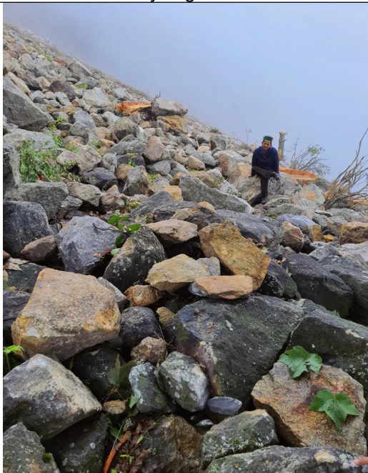
Fig.-8: Loose boulders in escarpment foot slope needs wire mesh draping and retaining .
